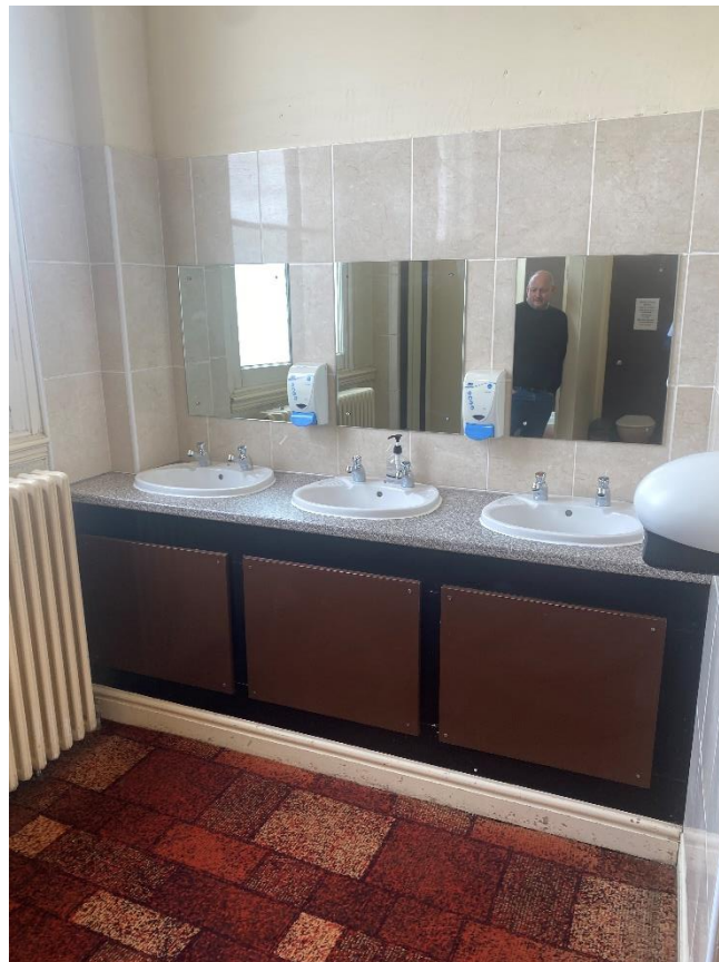
Figure 7 – Repair sanitary ware and undergo full redecoration in both gents and ladies' toilets
