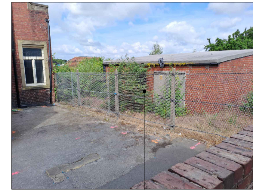
PHOTO 22 Wire mesh fence to NPG Sub-station
