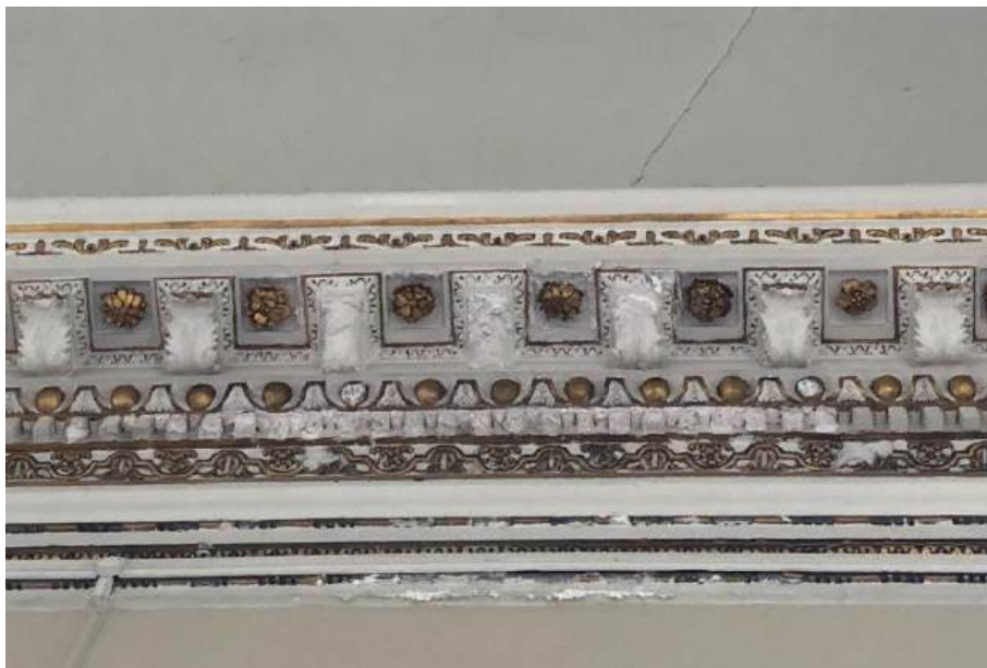
Figure 78. Deterioration of the cornice, Egg and Dart and Dental Blocks.
