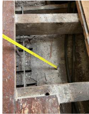
Figure 16. Pugging extending only partially over the edges of the ceiling.
