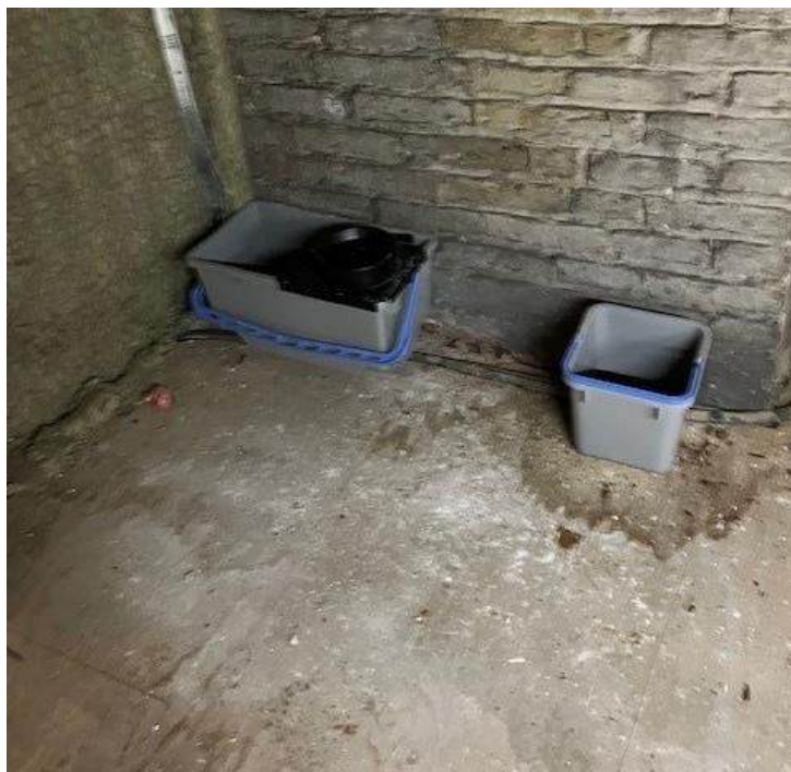
Figure 79. Water staining of the plywood surrounding buckets suggesting leaks in the area of the bucket.
