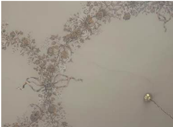
Figure 113. fractures found along the ceiling expanse.
