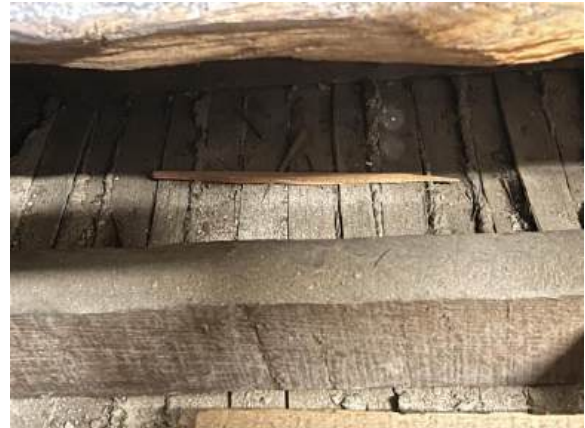
Figure 120. View of laths and nibs, laths are tight and nibs are sparce.
