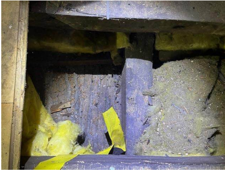
Figure 77. Location *5 showing the lath are spaced close together with minimal nibs present.
