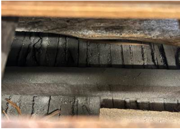
Figure 119. View of laths and nibs, many nibs are missing.
