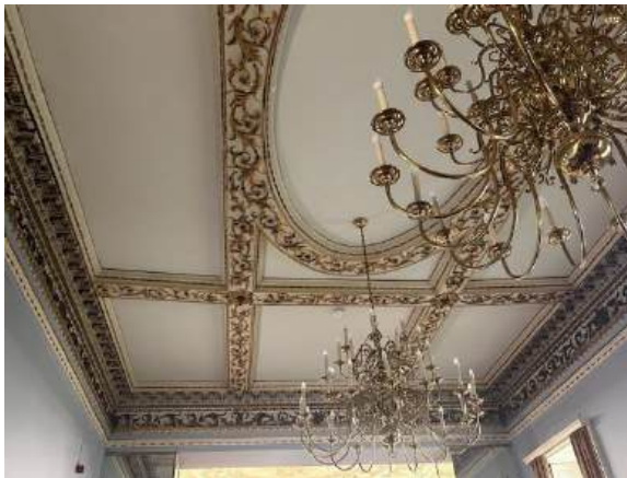
Figure 6. Ceiling bowing from East to West, visible on the beam.
