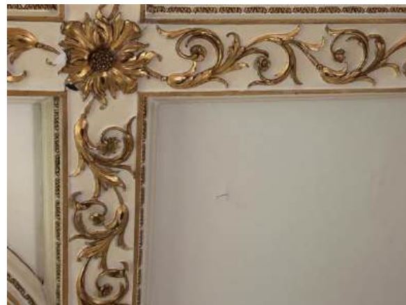
Figure 14. Minor delamination of skim coat and loss visible surrounding the enrichment.
