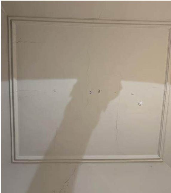
Figure 69. Fractures seen throughout ceiling expanse.
