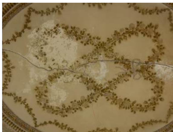
Figure 94. Multiple fractures run from the central significant fracture.
