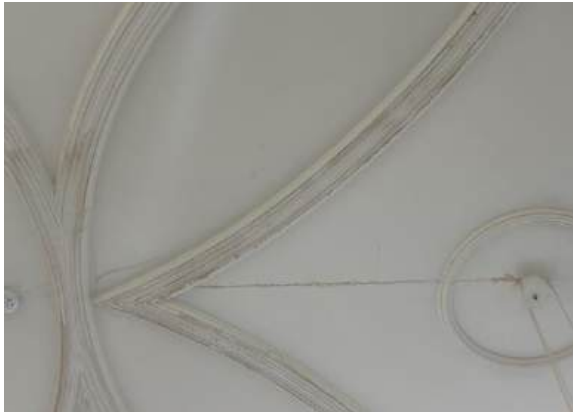
Figure 84. Hairline fracture on centre rose of ceiling.
