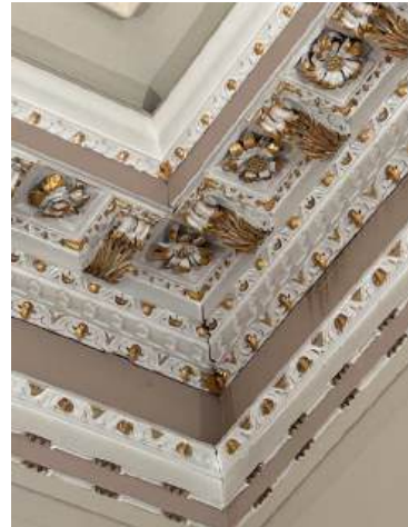
Figure 34. Cracks visible in the mitres.
