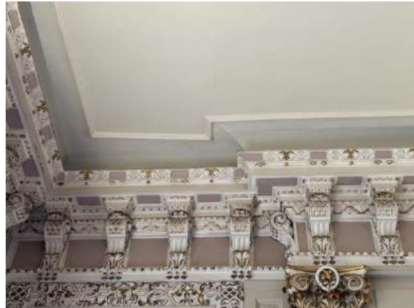
Figure 28. Minor deflection and evidence of a previous repair over the South wall cornice.
