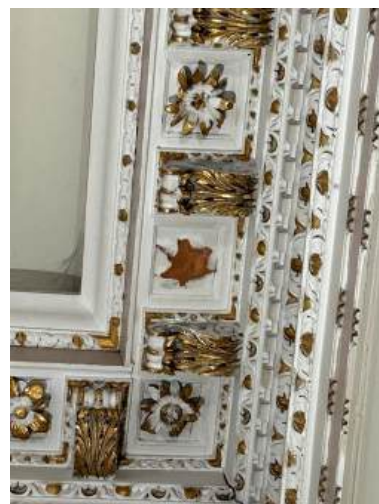
Figure 36. Missing embellishments throughout the cornice.
