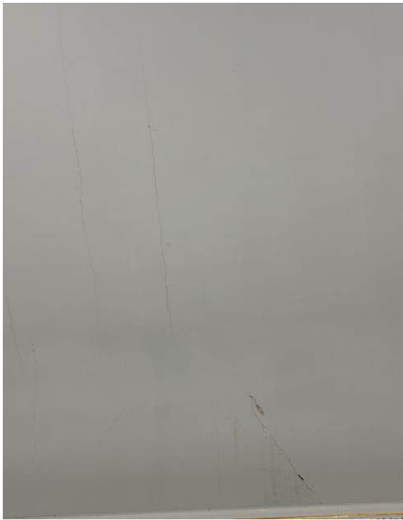
Figure 65. Multiple fractures running through ceiling.
