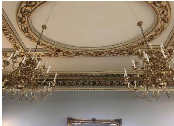
Figure 7. Bowing noted on West wall cornice.
