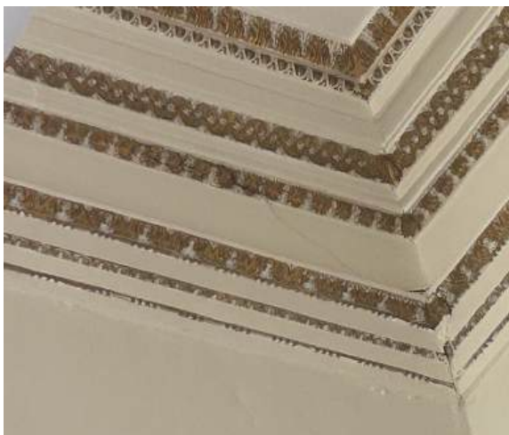
Figure 101. Fracture running along cornice.
