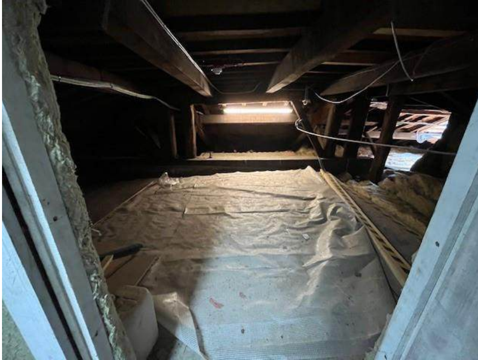
Figure 81. South End ceiling where plastic sheeting is present covering the walkway.
