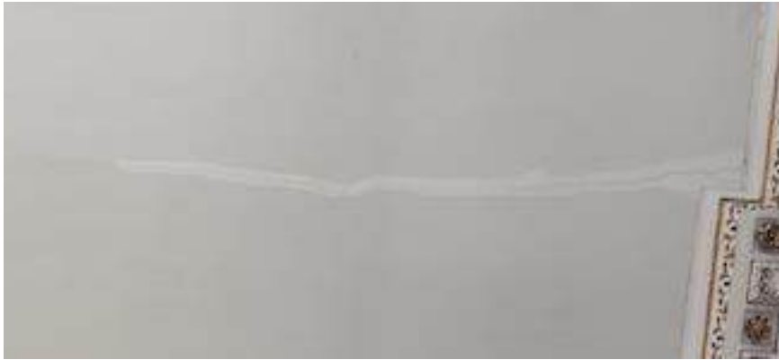
Figure 62. Fracture visible on the ceiling.
