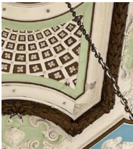
Figure 49. Area of loss on central border.
