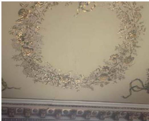
Figure 115. Fractures running through cornice.
