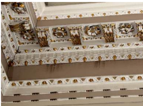
Figure 35. Possible water ingress visible on the cornice.
