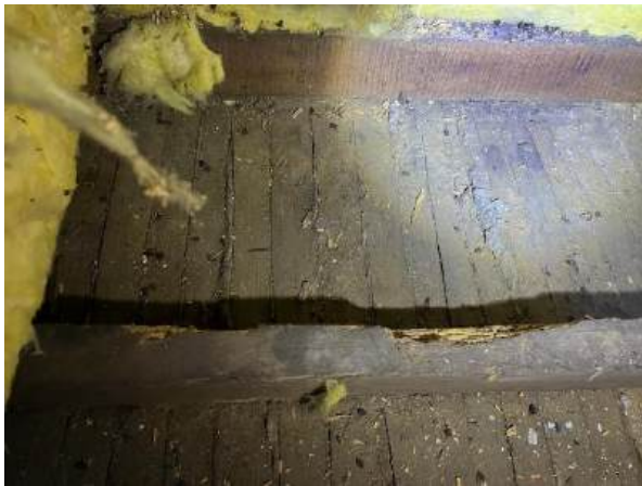
Figure 73. Location *1 lath to the North end of the Long Gallery, showing the spacing is too close together.
