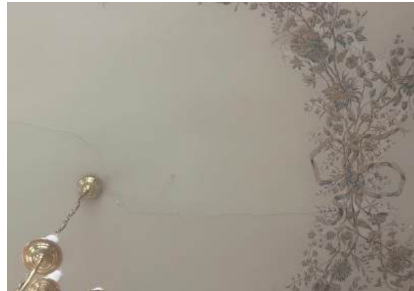
Figure 114. Fractures found along the ceiling expanse.
