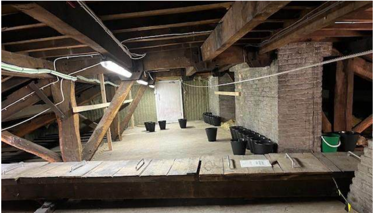
Figure 80. Location of the South End rainwater trough. Note the buckets placed along the chimney suggesting lead flashing leak and strategically placed buckets in the walkway.
