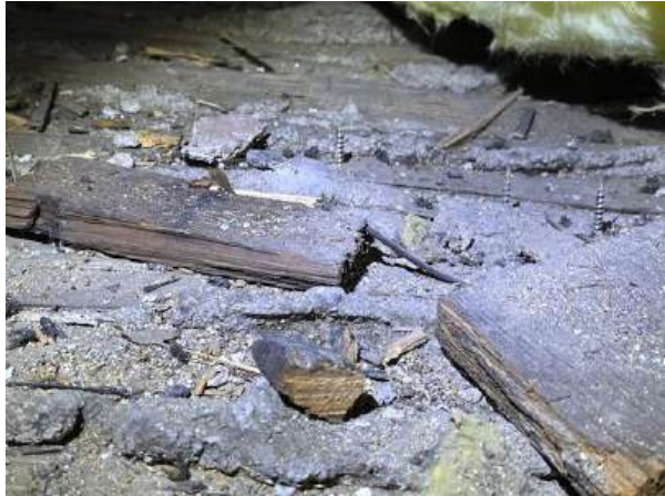
Figure 74. Screws through the lime plaster where the boards have been fixed to the ceiling. Note the lime plaster is still present in this area. Note the debris on the topside of the ceiling, located at *4 of the diagram.
