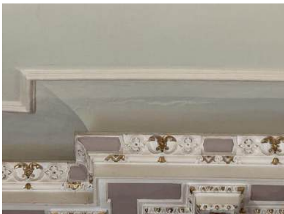
Figure 29. Previous patch repair visible.
