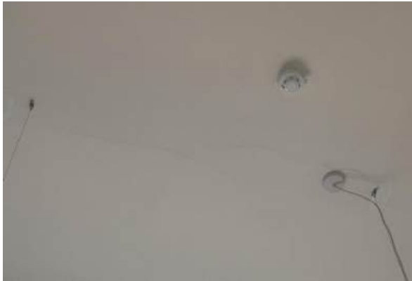
Figure 99. Fractures found running along the ceiling expanse.
