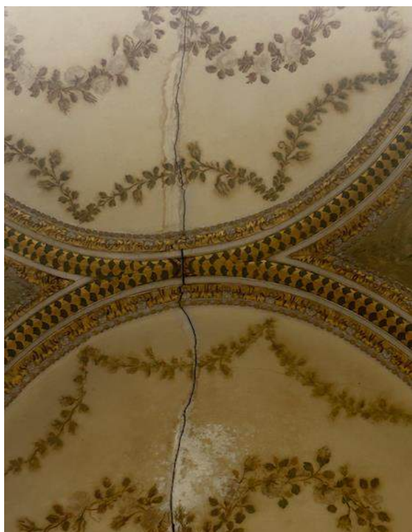
Figure 95. Possible water ingress observed around fracture.
