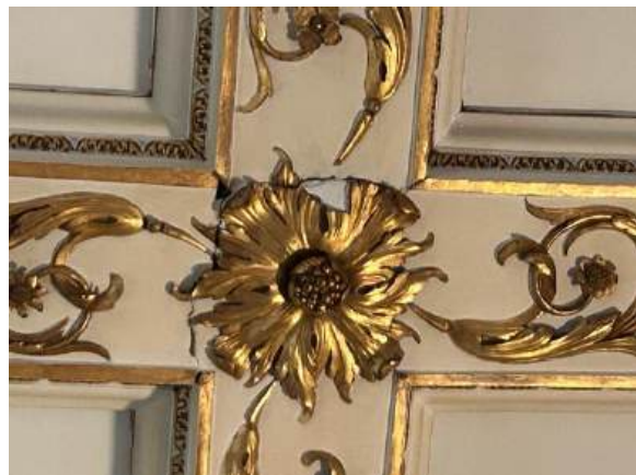
Figure 9. Fracture which could be a deliberate cut noted on multiple enrichments.
