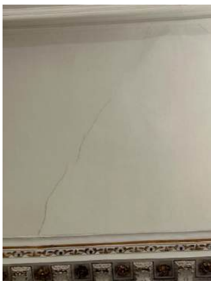
Figure 53. Hairline fractures noted throughout the ceiling.
