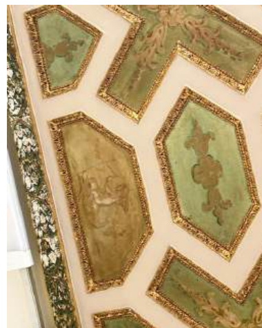
Figure 91. Fading noted on the painted decorative plaster border. Hairline fractures visible throughout.
