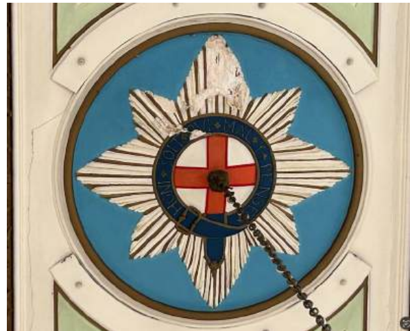
Figure 48. Area of loss in central rose.
