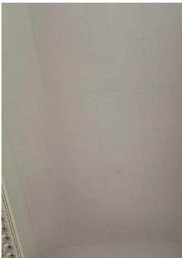
Figure 59. Plasterboard meeting seams visible on large expanse of the ceiling.
