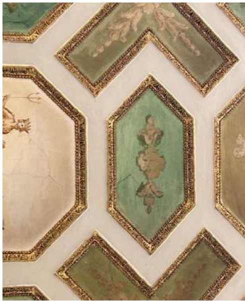
Figure 88. Hairline fractures found throughout the ceiling.
