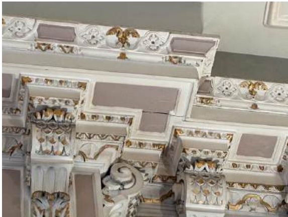
Figure 27. Fracture visible on the cornice.
