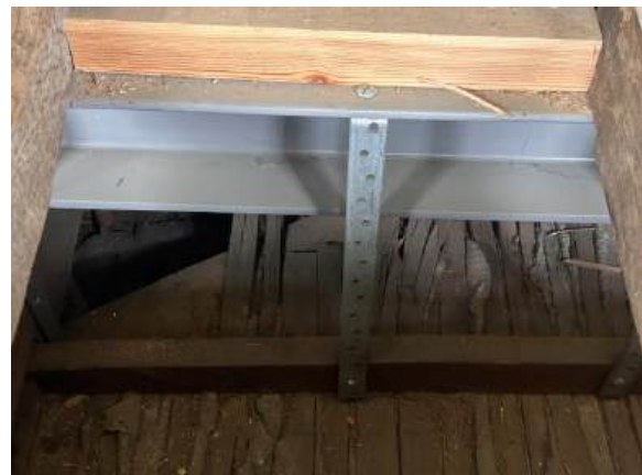
Figure 18. Later steel beam gives evidence of a second phase of intervention and stabilization. Bat straps are attached, connecting the plaster ceiling to the structural repairs above.
