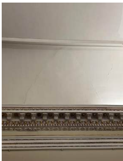
Figure 54. Shape of hairline fractures on North and South wall coves.
