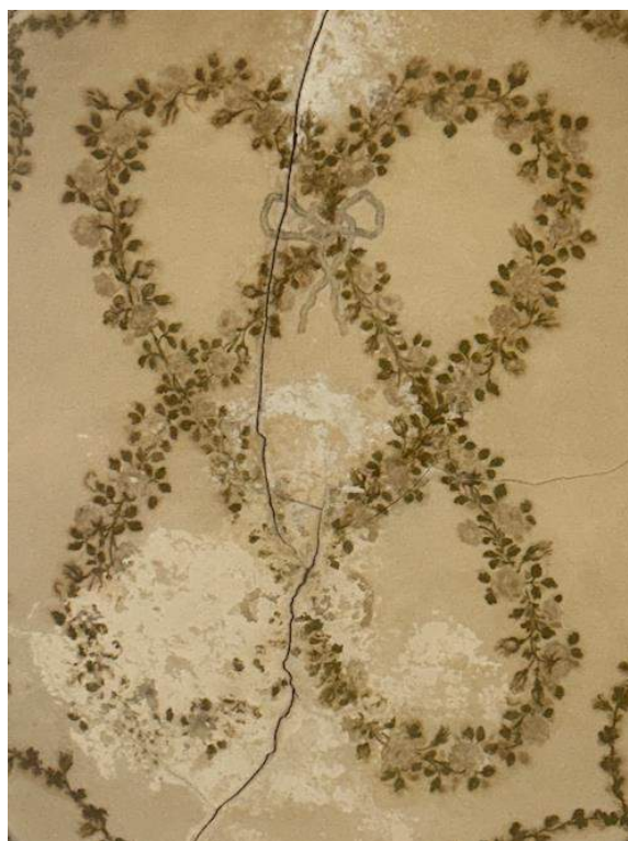
Figure 96. Paint loss, flaking, and fading seen throughout the painted ceiling expanse.
