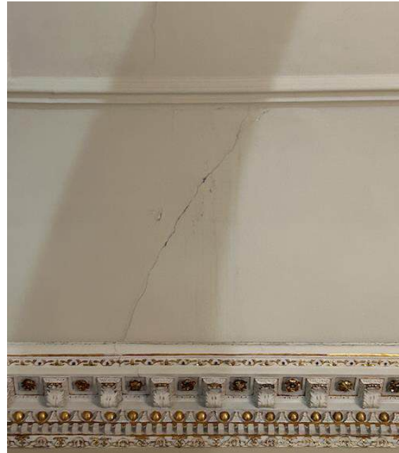
Figure 70. Fracture with loss and delamination and possible water ingress.
