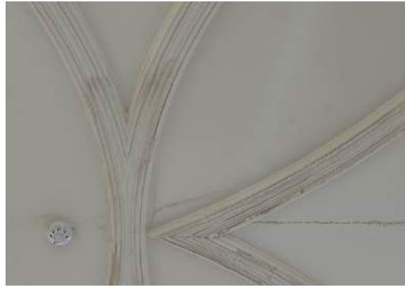
Figure 85. Possible water ingress marks near fractures.
