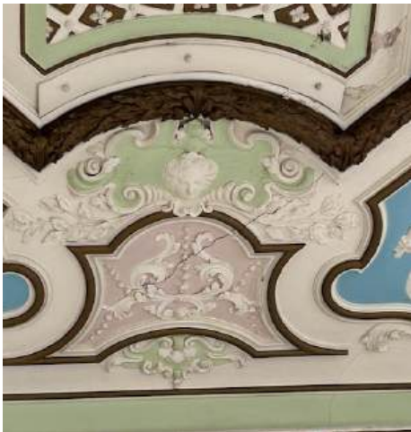
Figure 47. Hairline fractures visible throughout the ceiling.
