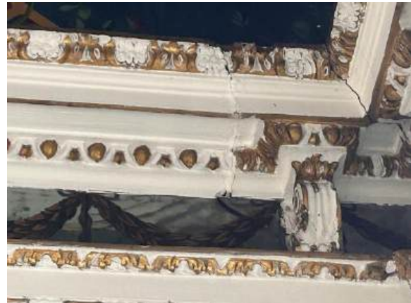
Figure 106. Crack running through cornice and causing a break in the mirrored frieze panel.
