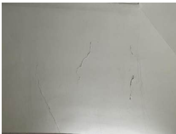
Figure 55. Fractures with delamination and potential water ingress or salts visible.
