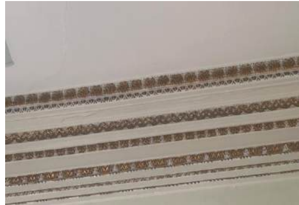
Figure 100. Fractures found along the cornice.
