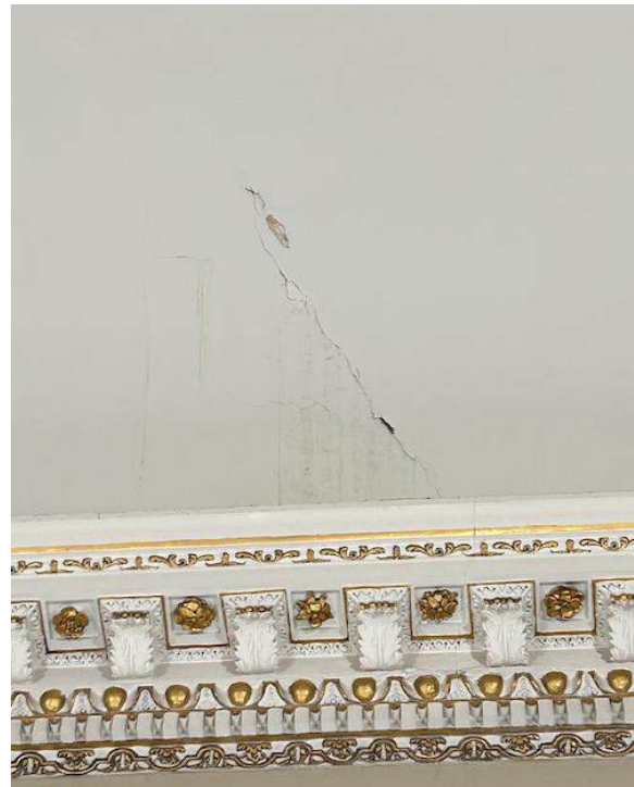
Figure 66. Fracture resulting in loss and possible ingress.
