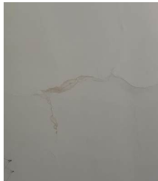
Figure 102. Possible water ingress visible surrounding fractures.
