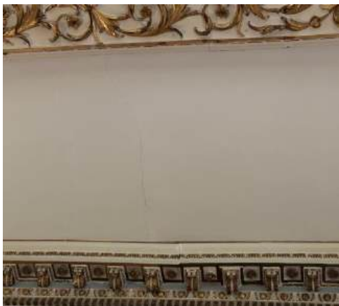
Figure 8. Hairline fractures noted throughout the ceiling.
