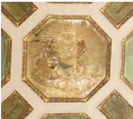
Figure 90. Possible water ingress resulting in paint loss and discolouration.
