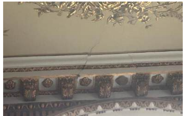
Figure 116. Fractures running through cornice.
