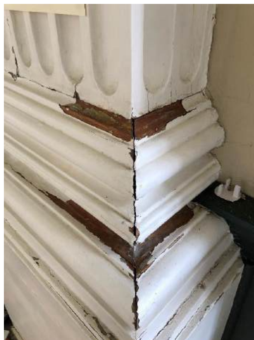
Figure 76. Flaking paint to the base of the column a result of water ingress causing the wood to swell and paint to delaminated.
