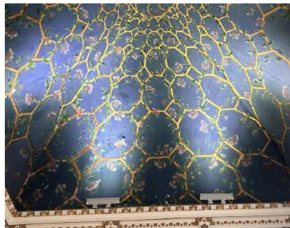
Figure 110. Loss, flaking, and discolouration visible.
