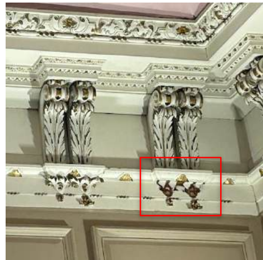
Figure 42. Multiple embellishments missing throughout the cornice.
