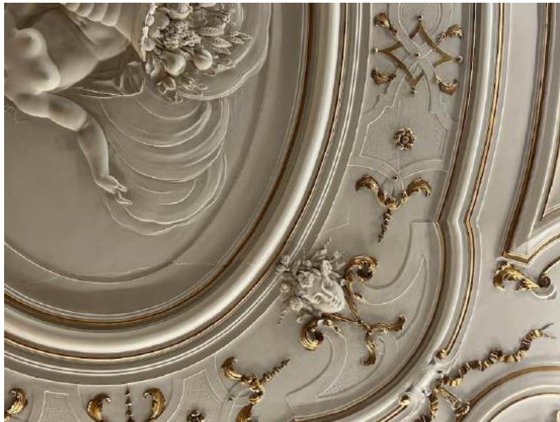
Figure 3. Image of hairline fracture running through the decorative plaster ceiling.
