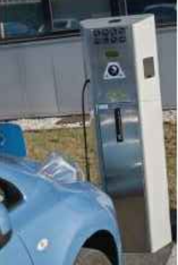
Typical Public Electric Vehicle Charging Point.
