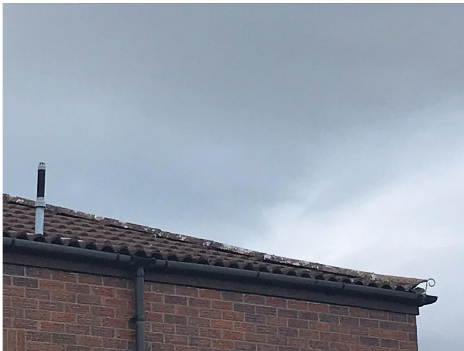
Photograph 12 – Raised and damaged ridge tiles ( TN7; Figure 1 ). Several instances recorded across buildings. Photograph taken of B1 .
