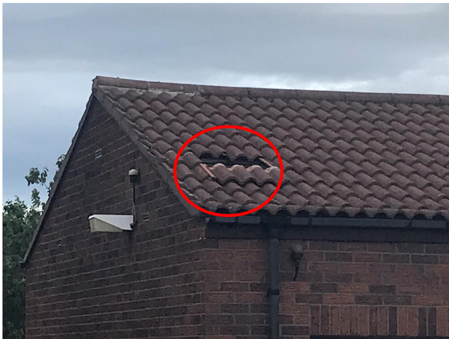
Photograph 9 – Missing tiles in pitched roof structure providing access to a potential loft void ( TN4; Figure 1 ). Multiple instances recorded across two buildings. Photograph taken of B1 .
