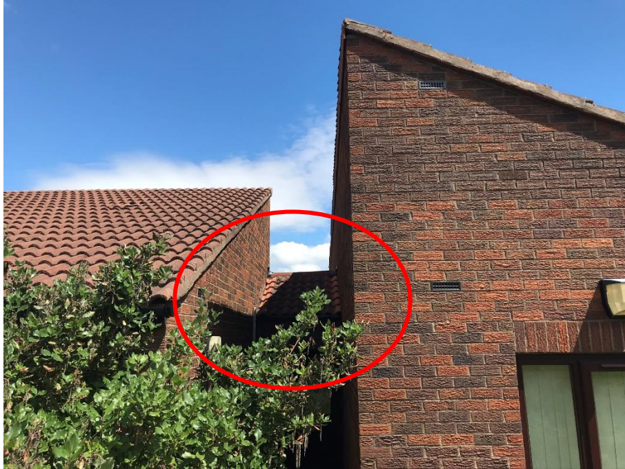
Photograph 14 – Instance of raised and damaged roof tiles amongst lifted lead flashing on a small rooftop (TN10; Figure 1). Photograph taken of B6.
