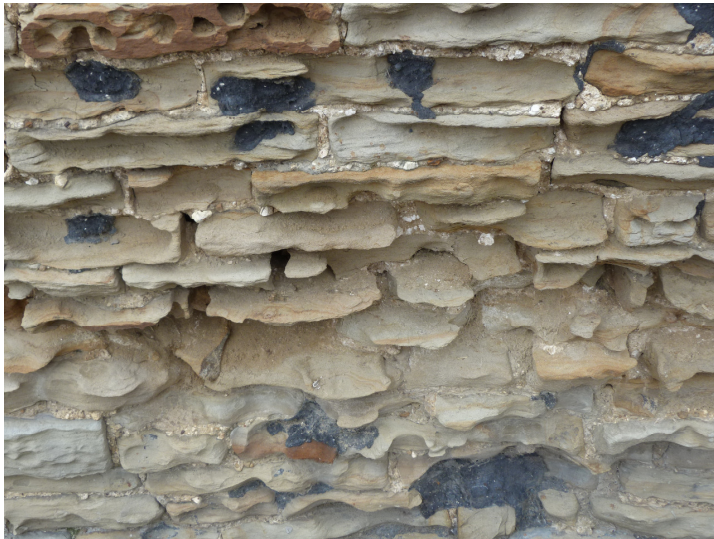
5. Typical stone erosion
