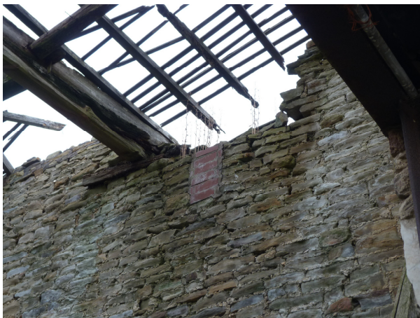
11. Collapse of south east elevation below eaves level
