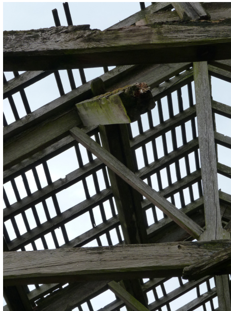
10. Collapse of decayed purlins
