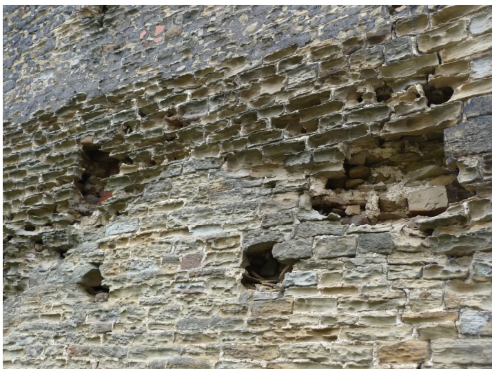
6. Significant erosion of north east gable
