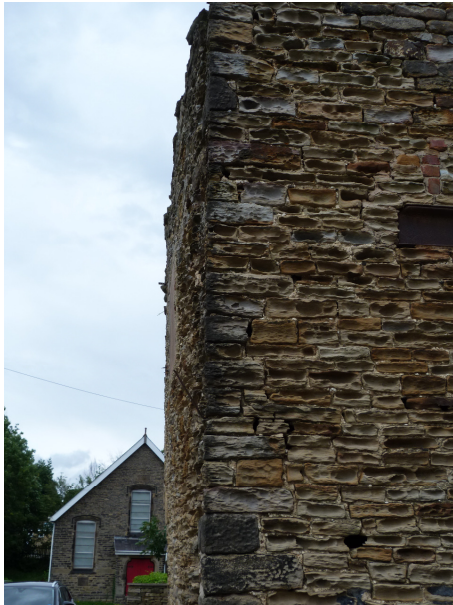
7. Lateral distortion of west elevation
