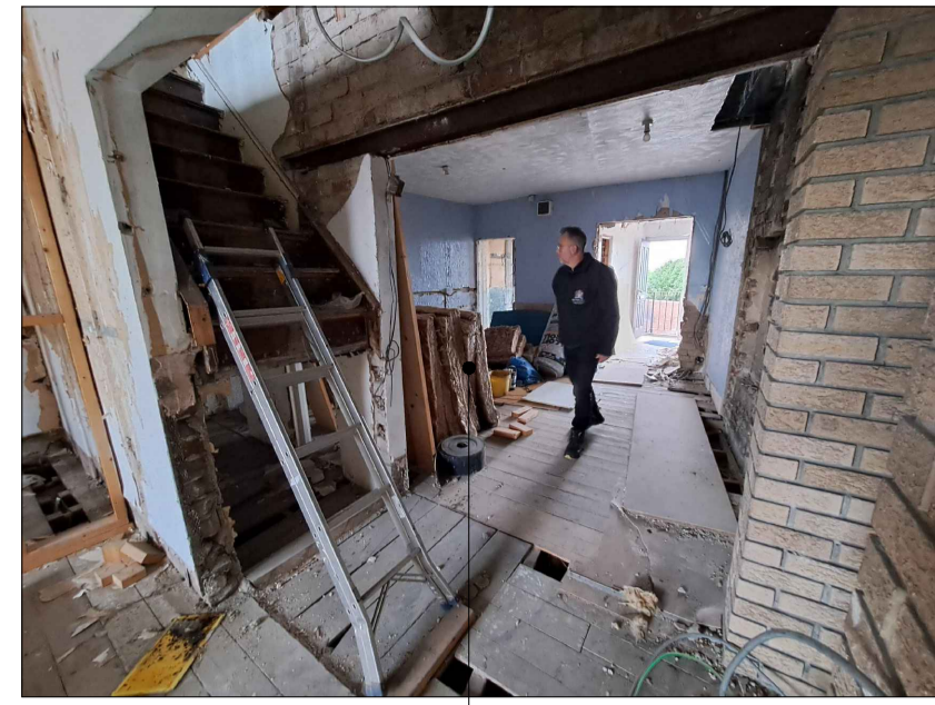
No. 301 at 1 st Floor level showing state of disrepair
