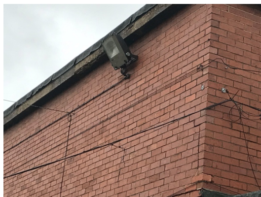
Image 6: Lifted felt on western side of Building 1
