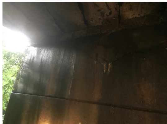
Image 4: Water running from cavities beneath the bridge piers
