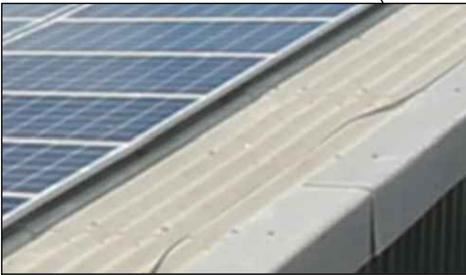
Cembrit Cemsix Fibre Cement (Natural Grey) Corrugated Sheets and 105.165kWp roof mounted solar PV
