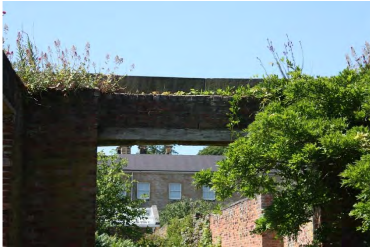
CRACKING TO BRICKWORK OVER WEST DOORWAY BUDDLEIA GROWING IN WALL HEAD
