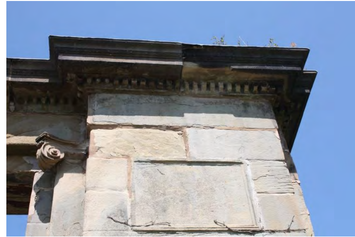
DISPLACED CORNICE TO EAST CORNER PIER
