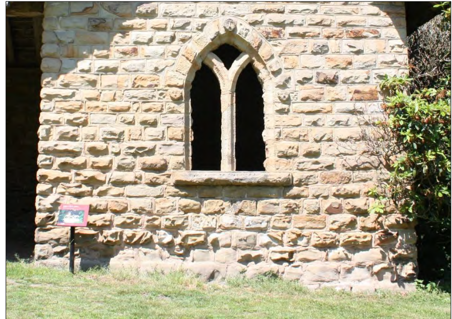
EROSION OF STONE FACE TO EAST GABLE
