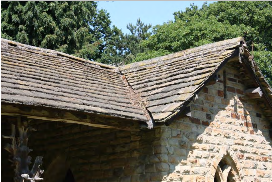
VALLEY GUTTERS CLOGGED WITH MOSS
