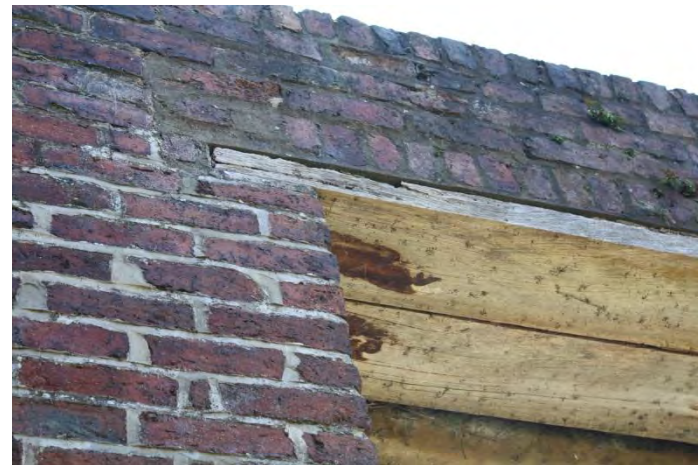
DECAY IN END BEARING OF INNER LINTOLS
