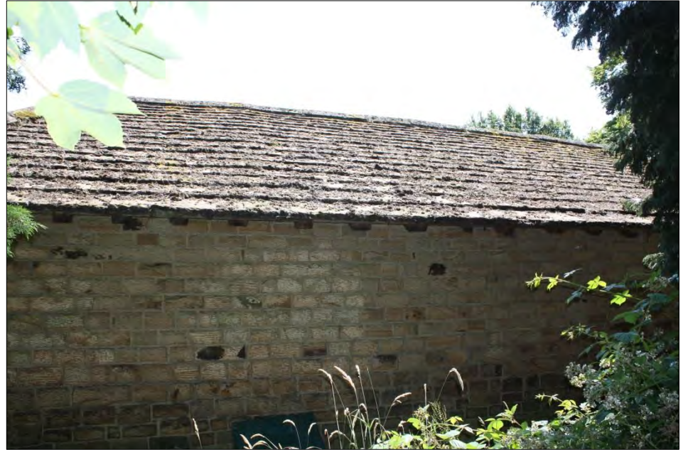
REAR ROOF SLOPE COVERED WITH MOSS
