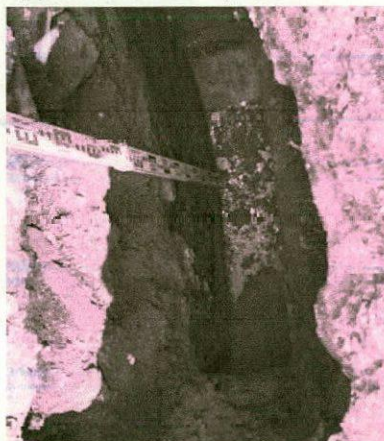
Plot 3: Approx. 0.70m made ground over what appears to be clayey sand.
