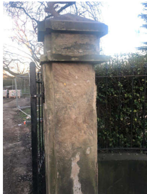
Fig 05. Right hand gate posts badly weathered and previously repaired.
