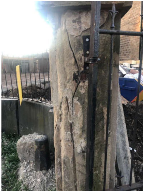
Fig 04. Left hand gate posts weathered and fractured from original iron hinge.
