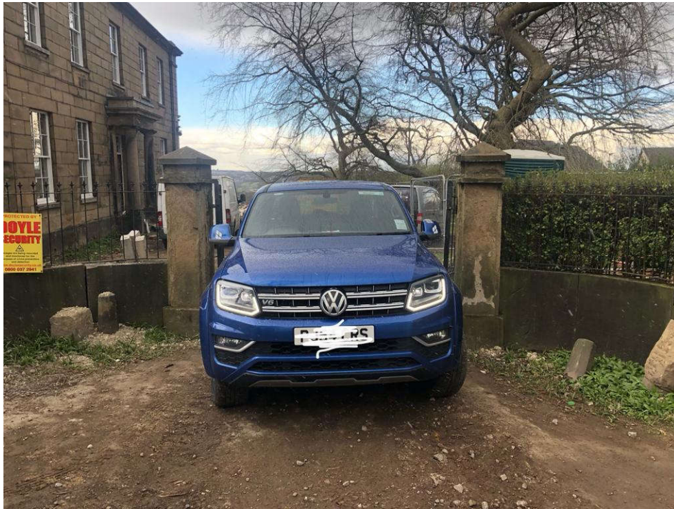
Fig 03. (Above) shows the existing entrance at less than 3.2m wide which is restrictive. Figs 04. and 05. Below show the condition of the existing stone gate posts which are badly weathered and fractured and require replacement to several components. These will be replaced using natural sandstone to match existing sections. Any components that can be salvaged, such as the cappings which appear to be in reasonable condition will be retained.
