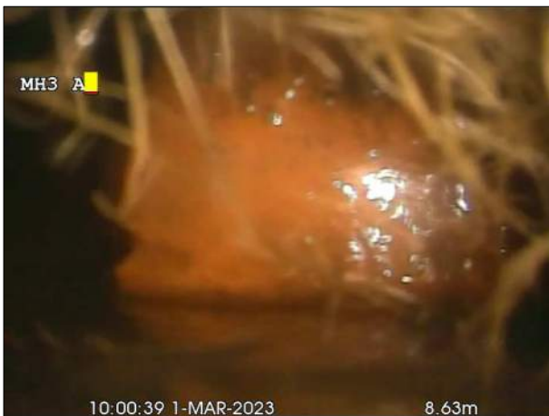
Photo: 3_6a, 00:00:00 7.5m, Obstruction, 80 % height/diameter loss
