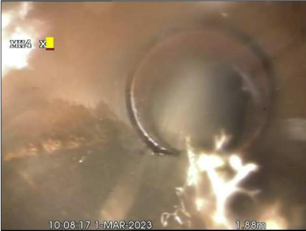
Photo: 42_4a, 00:00:00 1.9m, Joint displaced. Medium
