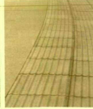
Hazard Warning Paving
