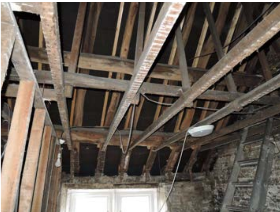
Roof over existing first floor bedrooms. Dry and weathertight. Specialist inspection recommended to check for fungal and insect attack.
