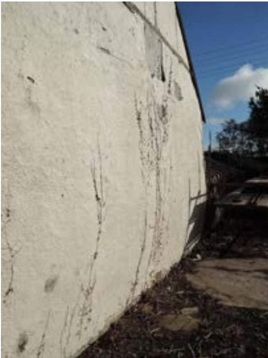
Severe outward bulge in same wall. Take down and rebuild
