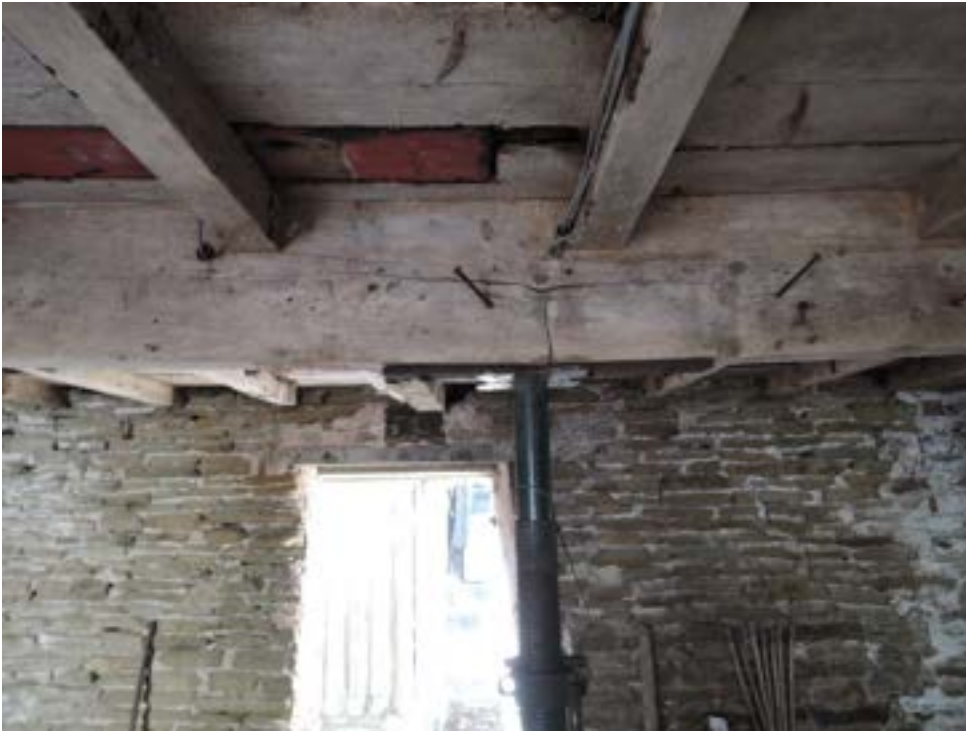
Small barn. Acrow prop to failed 1 st floor timber beam
