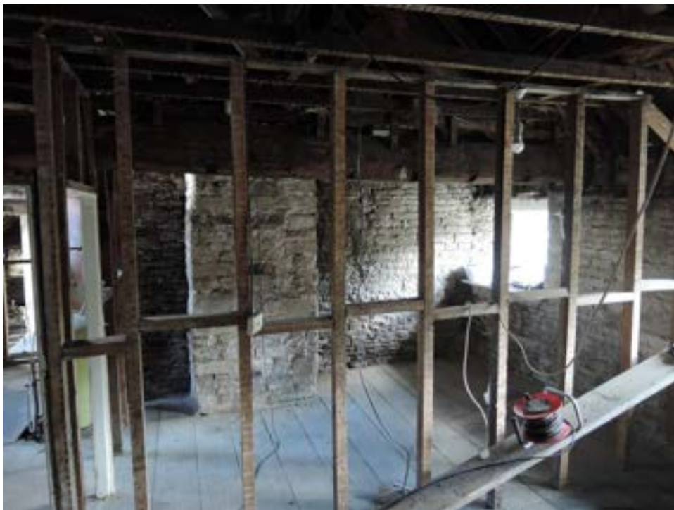
Stone flue from living room below (with cracked mantle). Terminates at ceiling and goes sideways into original chimney
