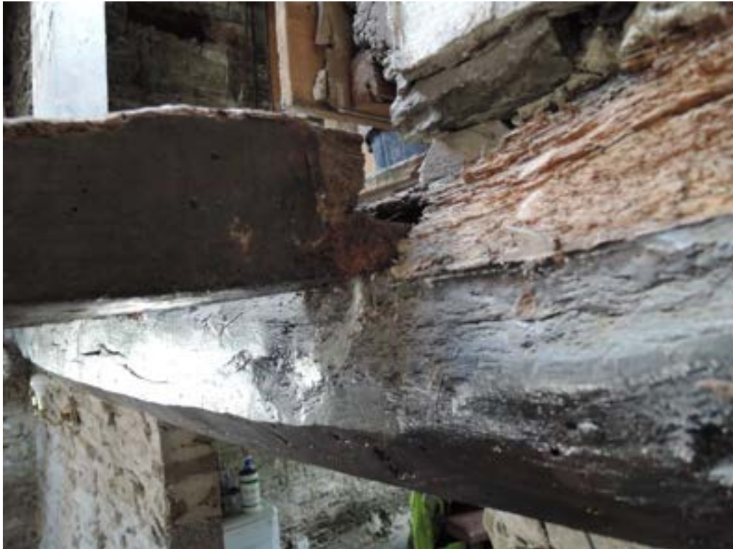
Joist end about to fail (several joists in this state)
