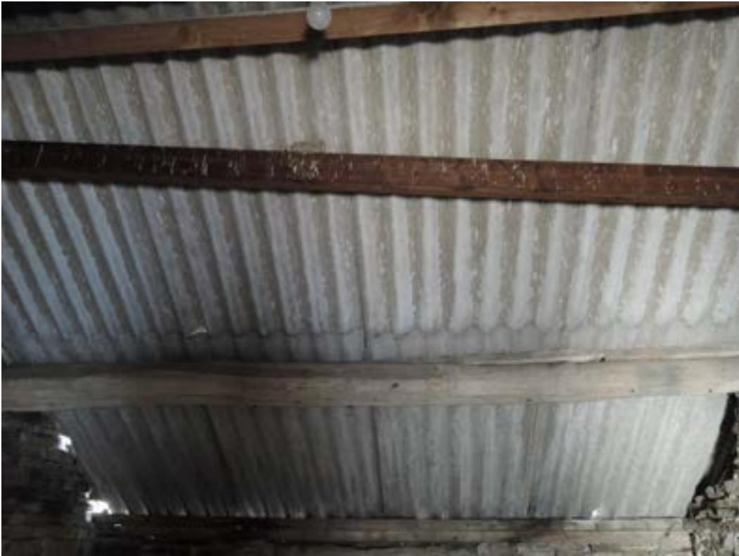
Roof. New rafters, purlins and covering required if being converted for habitation
