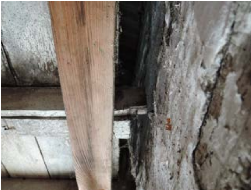
Wall has drifted out circa 75-100 mm completely releasing and abandoning first floor joist ends.
