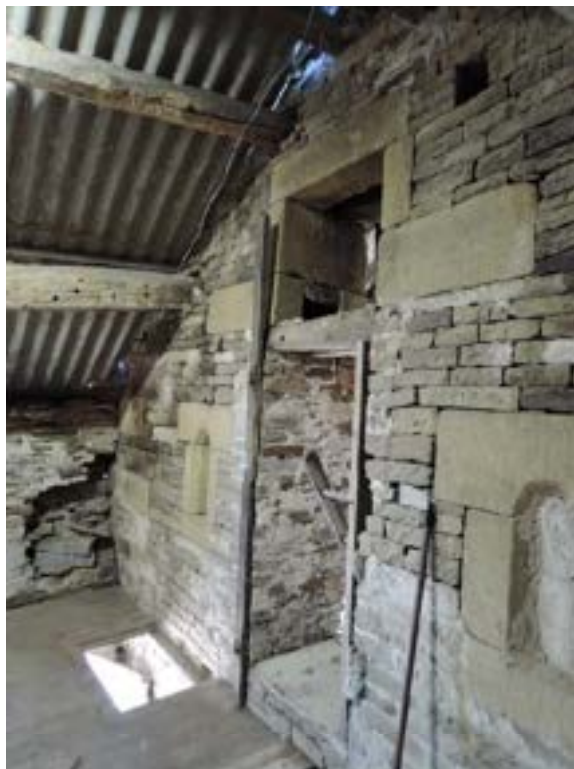
1st floor small barn. Pronounced lean of gable wall of large barn. Take down and rebuild
