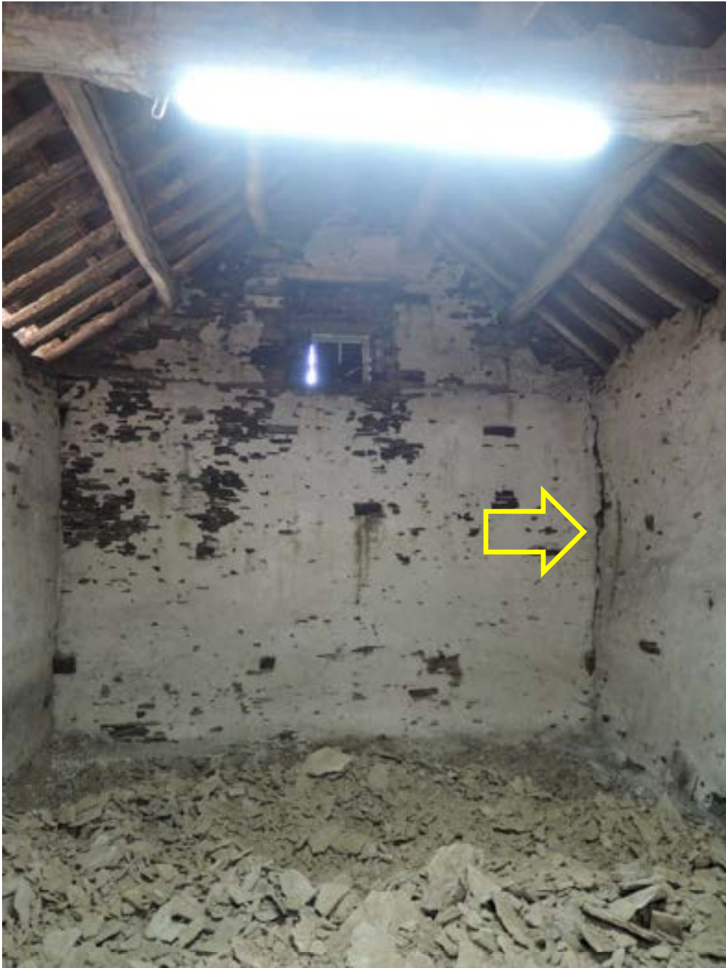
Large barn south gable. Bulge and crack arrowed where flank wall has released. Local dismantling and rebuilding recommended. Add this to the 'take down and rebuild' recommendation of the outward bulging gable (page 22). This picture is the inside face of the south gable
