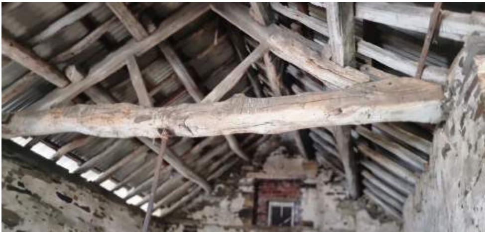
Internal Image of part of the Roof Structure in one of the Listed Barns
