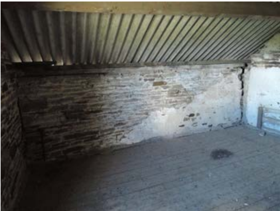
Corner cracking in wall junction indicating outward wall lean and lack of tying in
