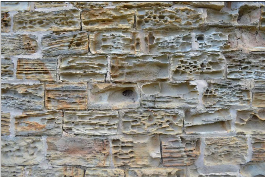
Figure 10: Detail of eroded masonry and cement pointing on the north-west gable.
