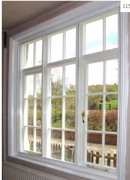
Plate 13 - Single glazed timber casement with secondary glazing incorporated (Historic England)
