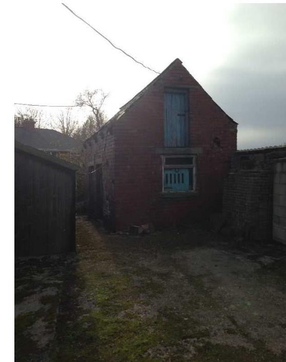
Photograph 12: View looking immediately south along the western boundary of the site. Note, the double storey outbuilding, in disrepair.
