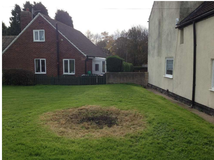
Photograph 7: View to the rear of the farmhouse building, looking south. An area of bare ground noted within the lawn. Map records indicate the previous location of a mature tree.
