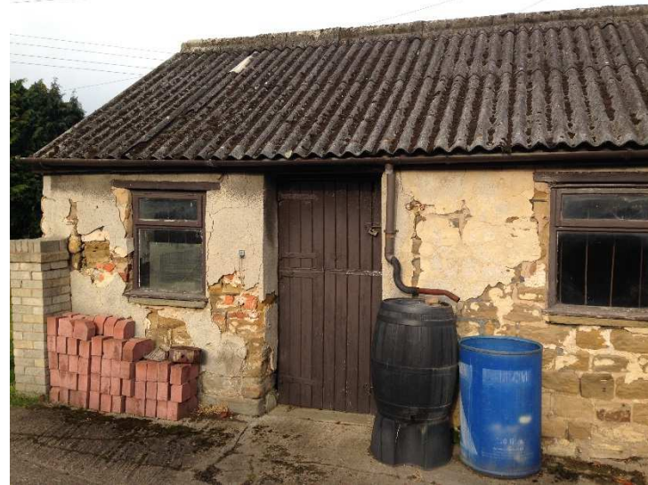
Photograph 2: View looking north towards an outbuilding situated in the north western extent of the site. The building was observed as largely empty with an empty drum and water butt outside. Potential corrugated asbestos roofing identified on the building.
