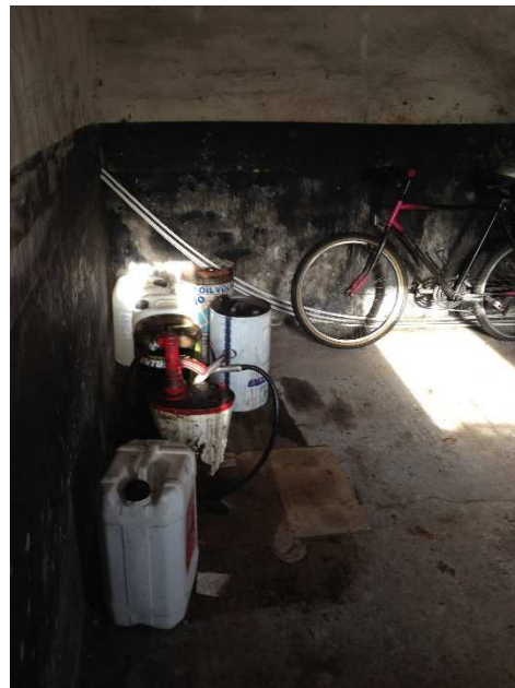
Photograph 4: View looking into the disused stable (photograph 3). Note, car oil and hydraulic oils and grease. The ground floor slab within the building was recorded as being in good condition with no obvious cracking.
