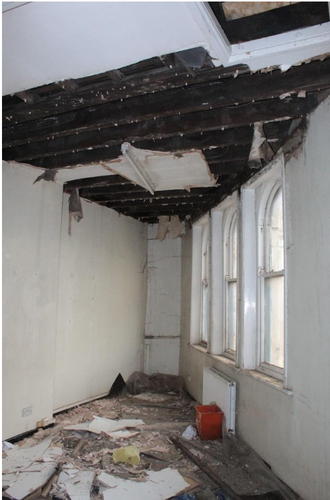
Fig 13. The collapsed ceiling under the flat roofed section of the central block.
