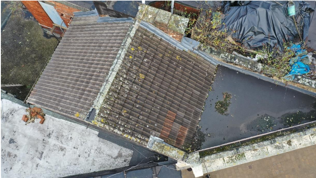
Fig 12. The roof of no. 34 Eldon Street (taken by drone from the south).
