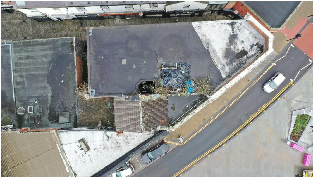
Fig 14. The roof of all three Haral Building roofs (the flat roof of the block containing no's 36 & 38 Eldon Street and no's 39 & 41 The Arcade is the large flat roof top and central).
