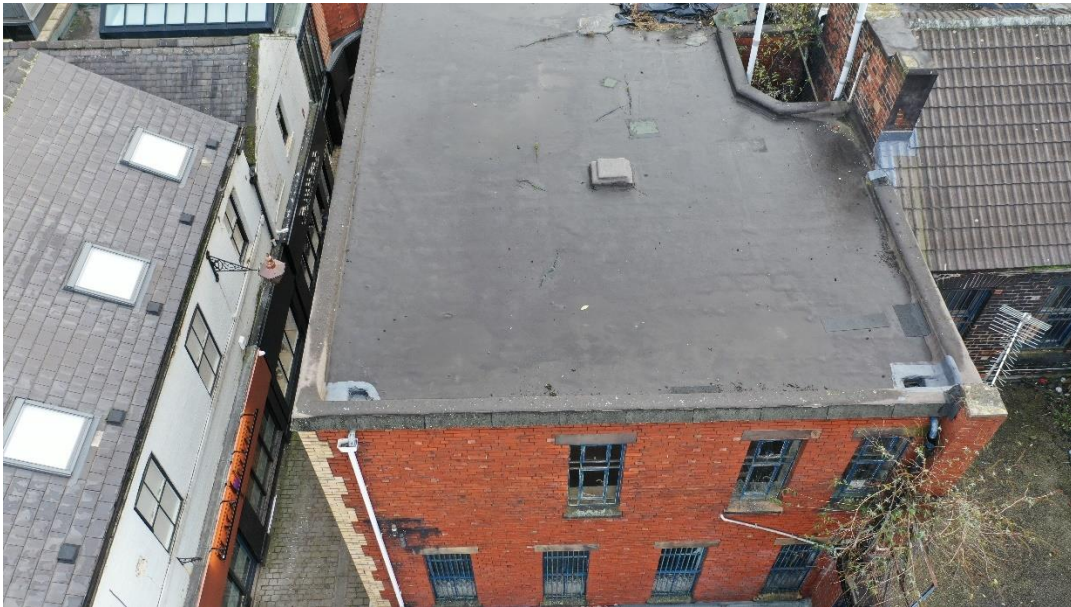
Fig 15. The roof above 39 & 41 The Arcade. Note the fresh paint around the outlets and the quantity of cracks in the bitumen/asphalt roof covering (taken by drone from the west).
