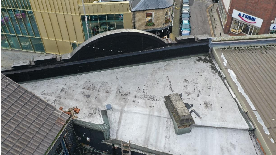
Fig 11. The roof of no. 32 Eldon Street (taken by drone from the north).
