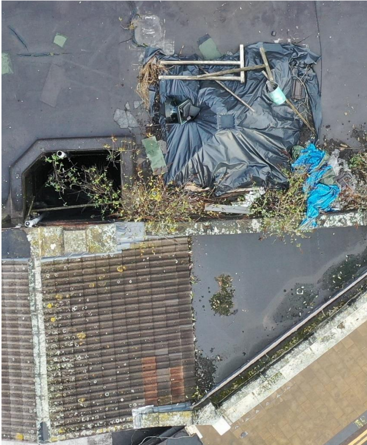
Fig 20. The glazed lantern has been temporarily covered with black visqueen sheeting.
