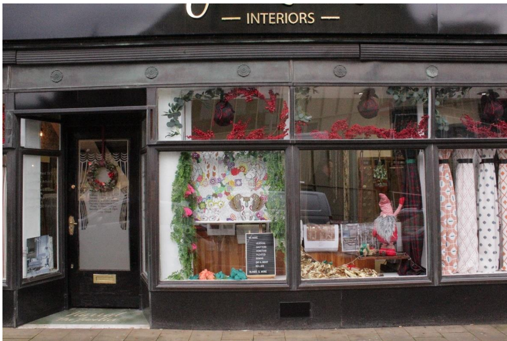
Fig 28. Distortion of the bronze window to the RHS of the Prisco's entrance (32 Eldon Street).
