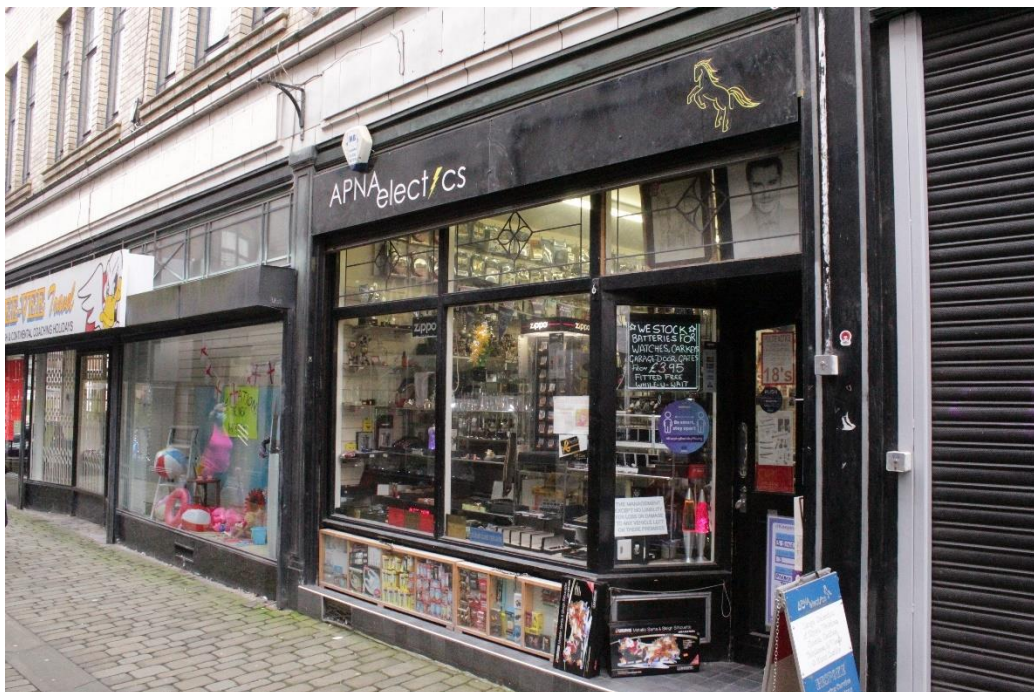
Fig 29. The historic bronze shopfront (far left) on the back of no. 36-38 and the bronze clad pilaster between this shopfront and that of no. 41 The Arcade which is a modern softwood replacement.
