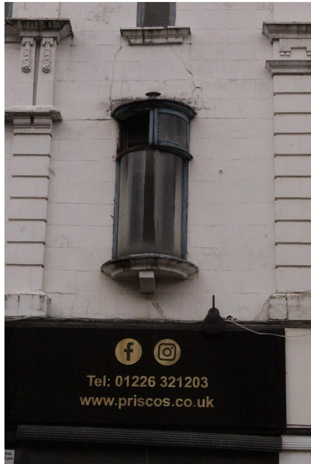
Fig 23. The cracked faience blocks between the narrow first and second floor windows.
