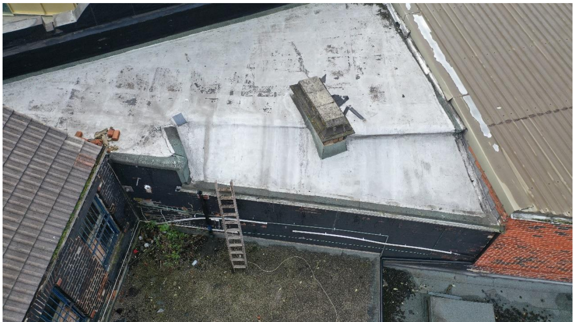
Fig 27. The rear elevations of no. 32 and no. 34 blocks which have been painted with black masonry paint.
