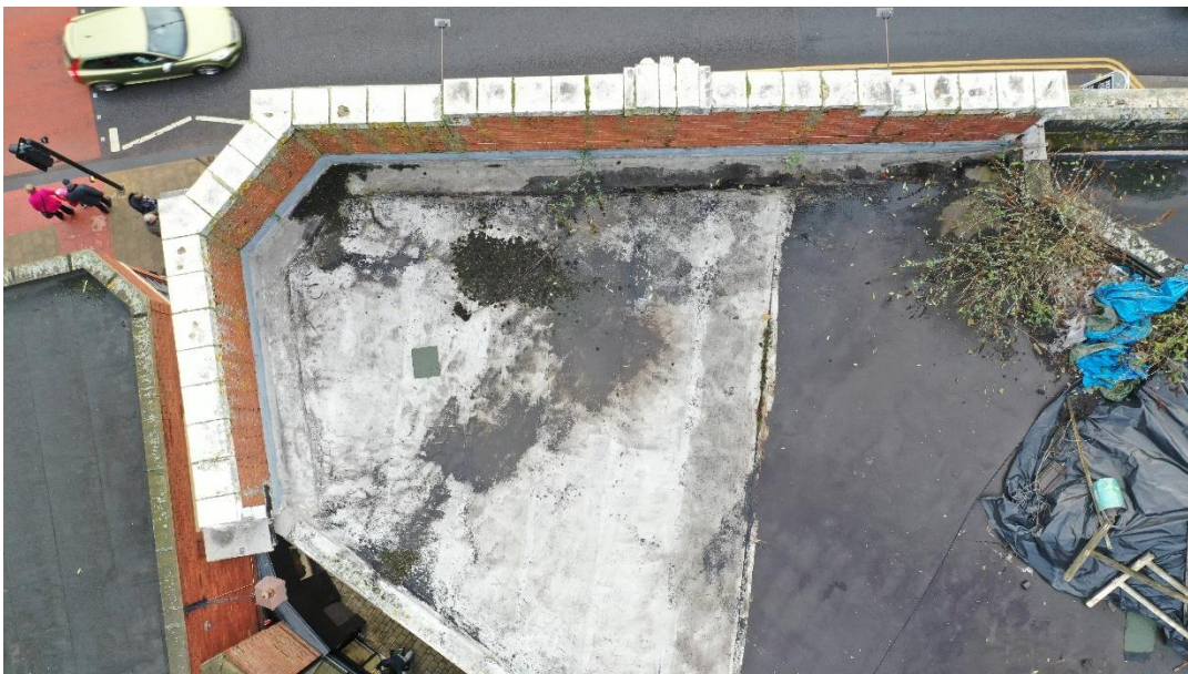
Fig 16. The roof above 38 Eldon Street. Note the lack of a flashing along the faience parapet and the presence of vegetation and pitting (taken by drone from the north – looking towards Eldon Street).
