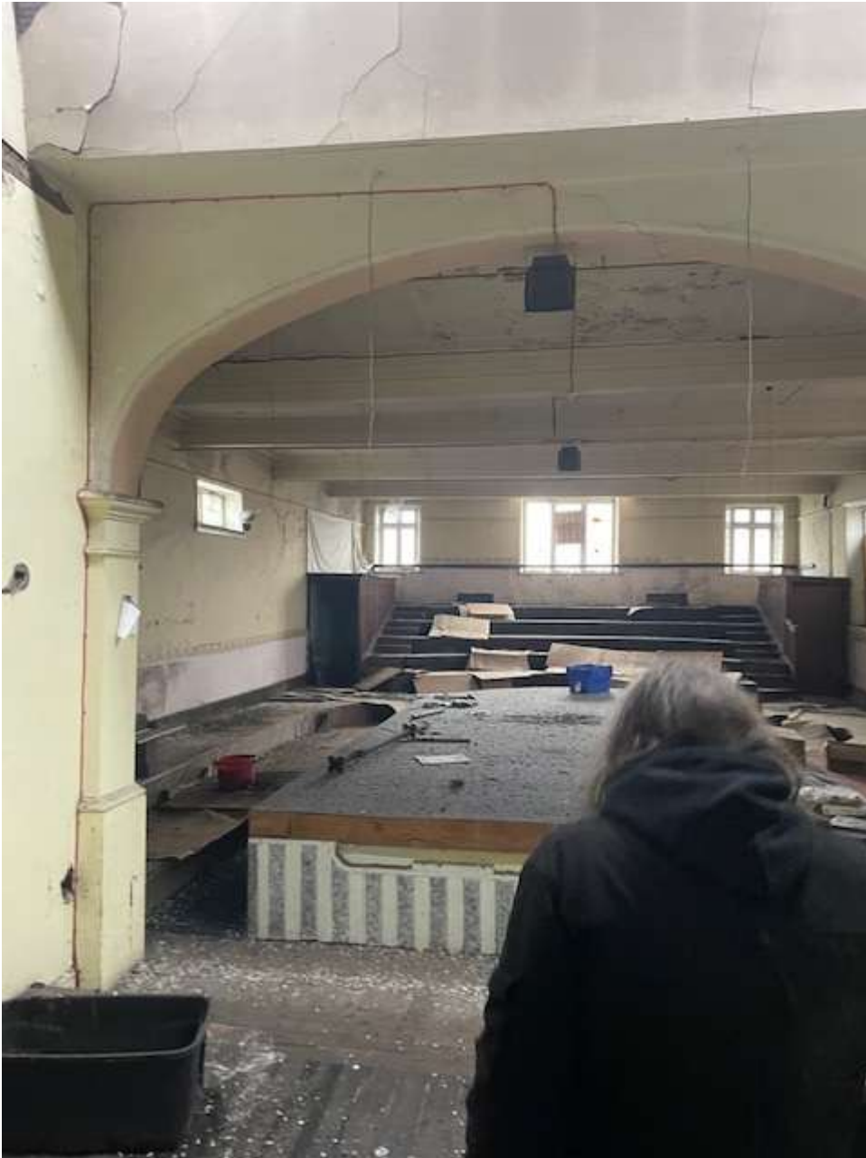
Upper floor front room propped
