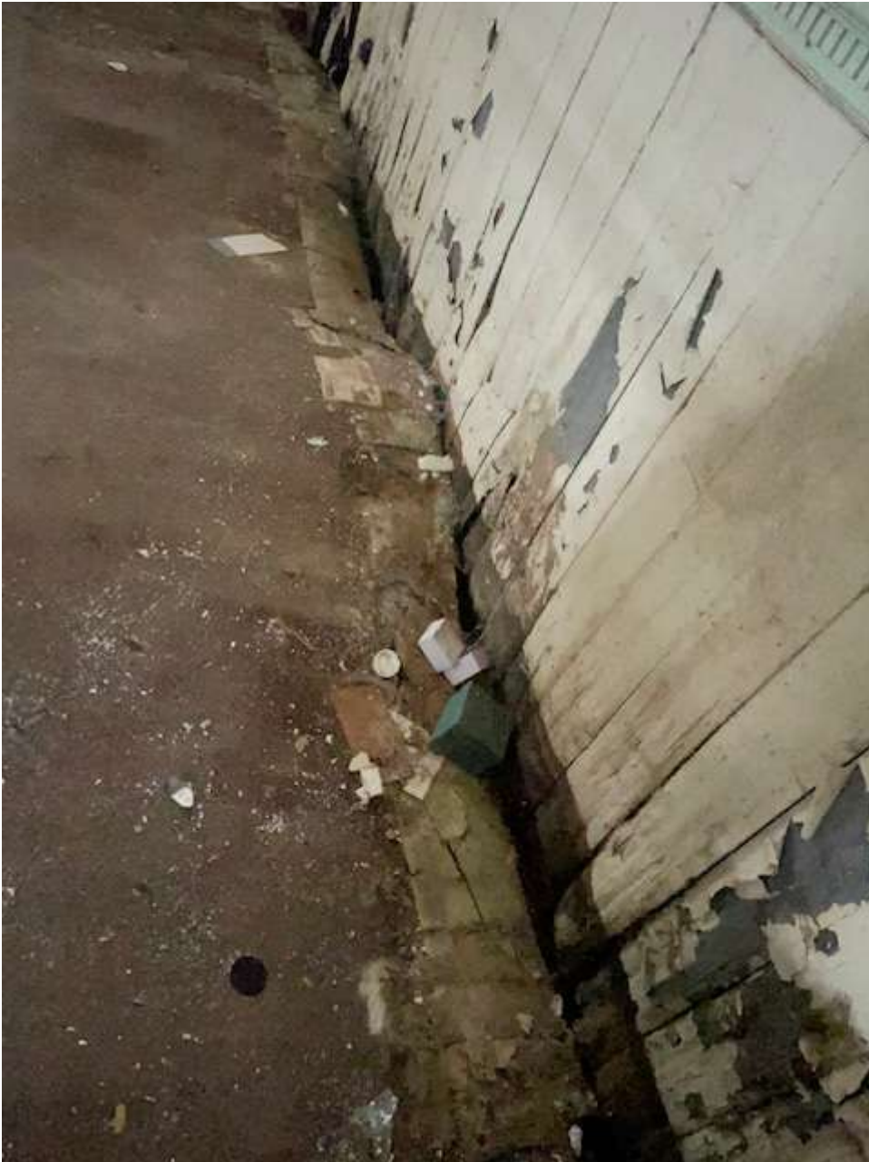
Ground floor front room. Floor falling away due to subsidence
