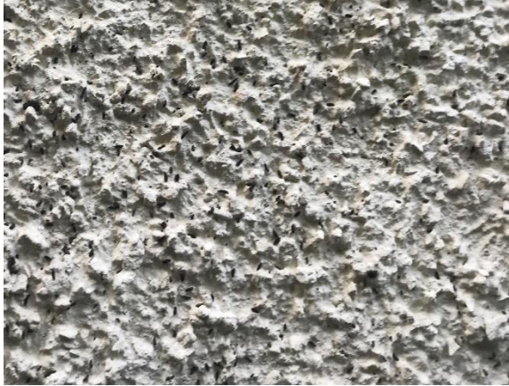
Bat droppings on an external wall
