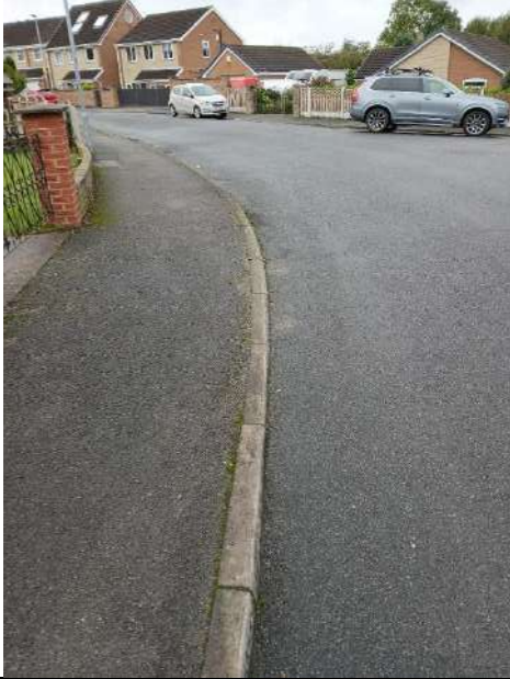
Minor footway damage.
