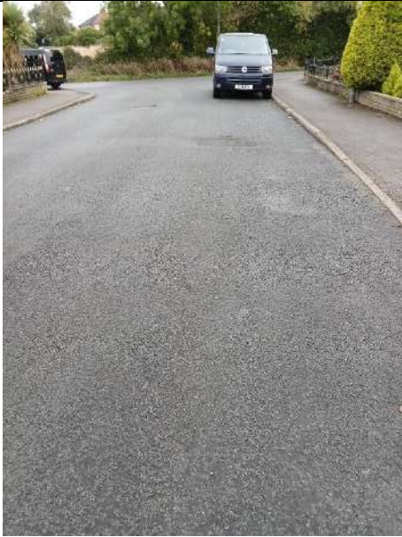
Minor carriageway damage.
