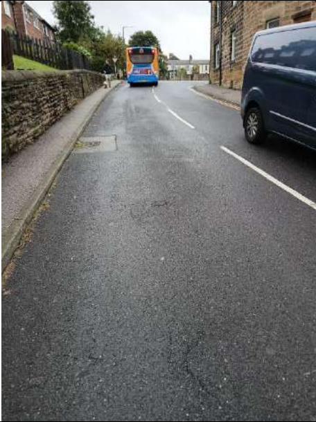
Minor carriageway surface course damage.
