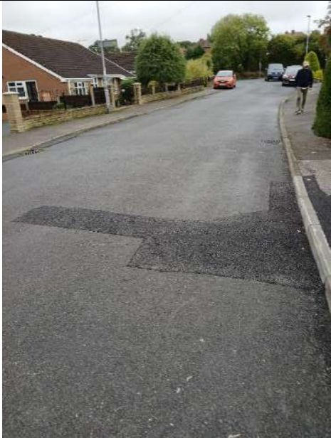
Carriageway and footway scarring.
