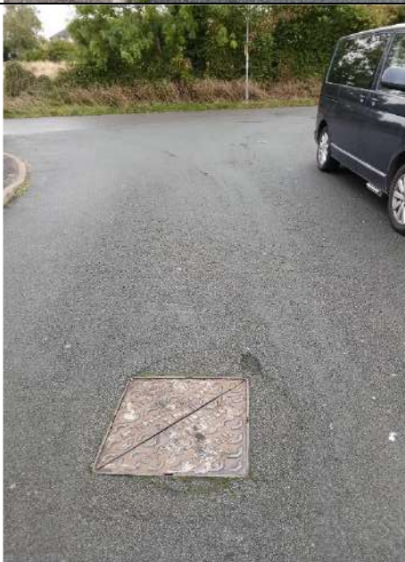
Minor carriageway surface course damage.
