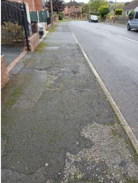
Footway surface course deterioration.
