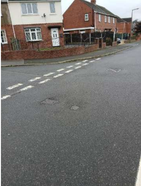
Carriageway surface course damage.
