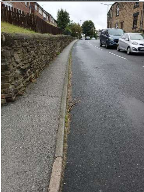
Minor kerb damage.
