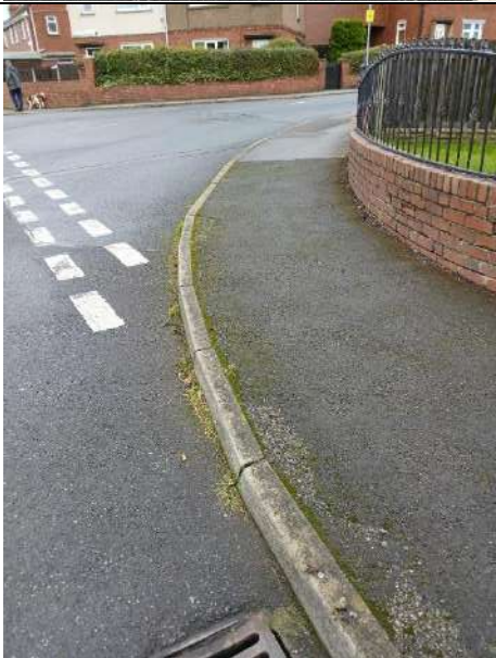
Carriageway scarring. Footway scarring. Footway minor surface course damage.
