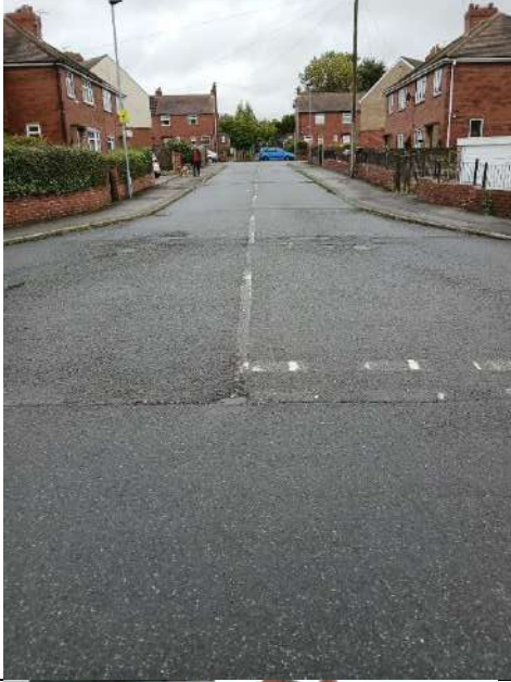
Carriageway surface course damage.
