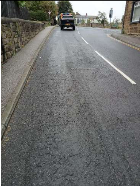
Carriageway surface course deterioration.
