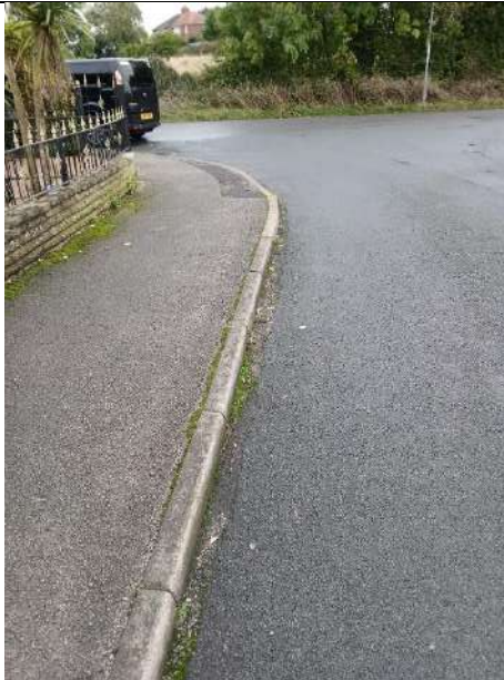
Minor carriageway damage. Footway scarring.
