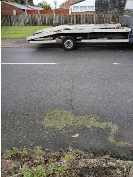
Carriageway surface course cracking.
