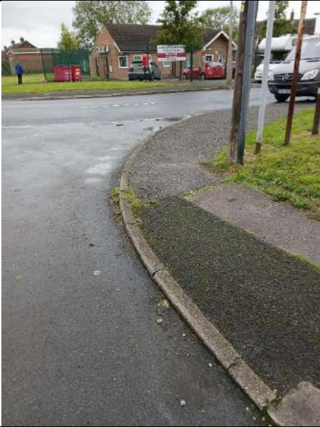
Footway scarring. Kerb damage.
