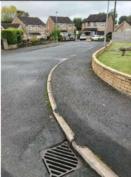
Footway and carriageway scarring. Kerb damage.
