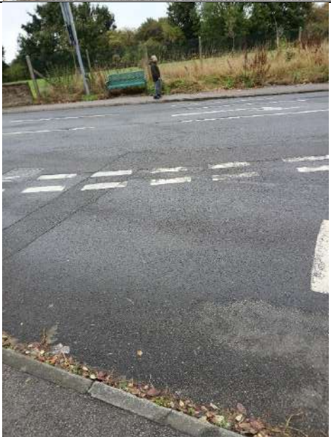
Carriageway scarring. Lining is wearing.
