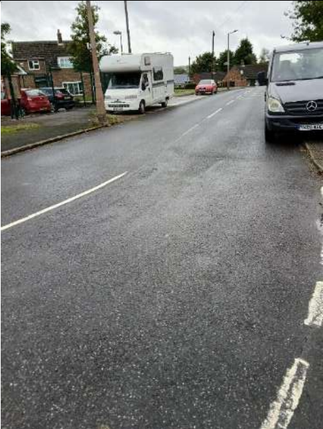
Minor carriageway surface course damage.
