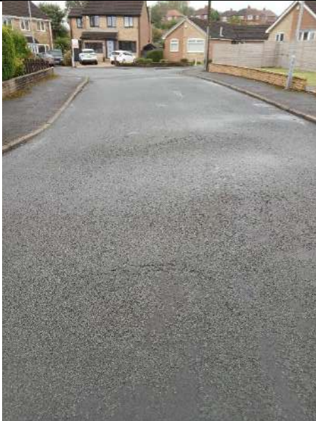
Surface course cracking. Uneven levels.
