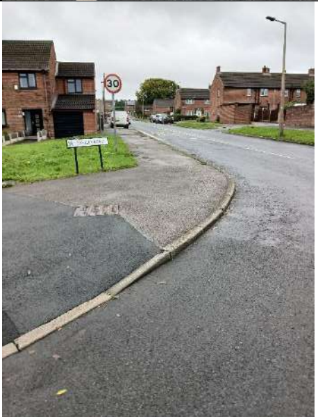
Kerb damage. Carriageway surface deterioration.
