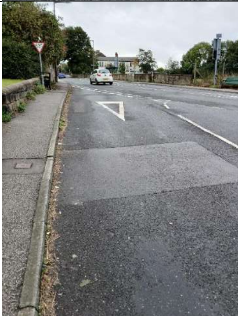
Carriageway scarring. Kerb damage and scarring.
