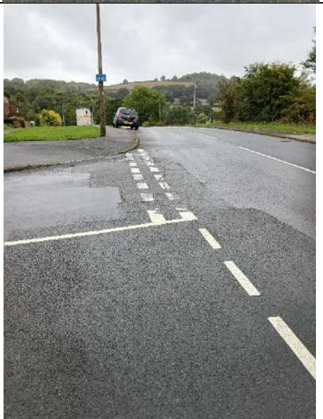
Scarring. Surface course deterioration.
