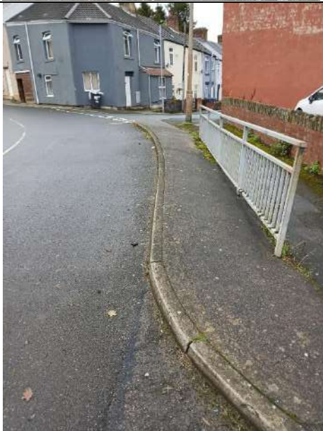
Footway / concrete verge cracking
