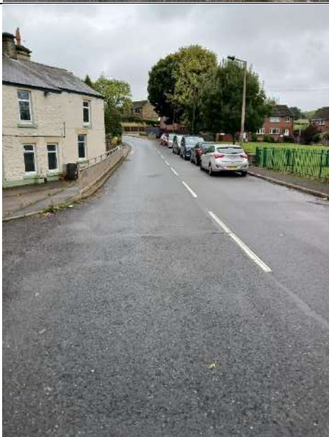
Minor carriageway surface course damage.
