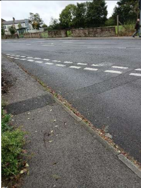
Footway / carriageway scarring.
