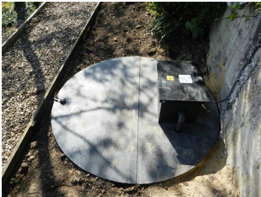
Installed Sewage Treatment Plant
