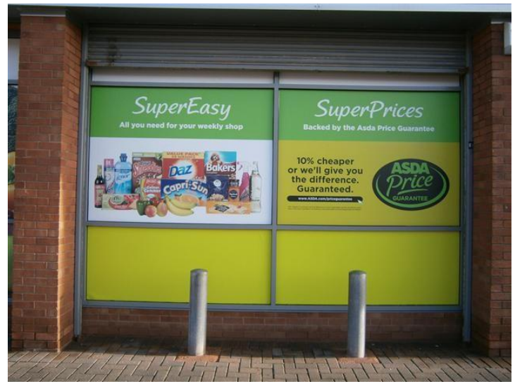
Roller shutter No. 8 - Concealed
