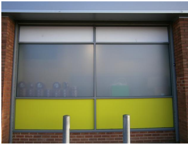
Roller shutter No. 6 - Concealed
