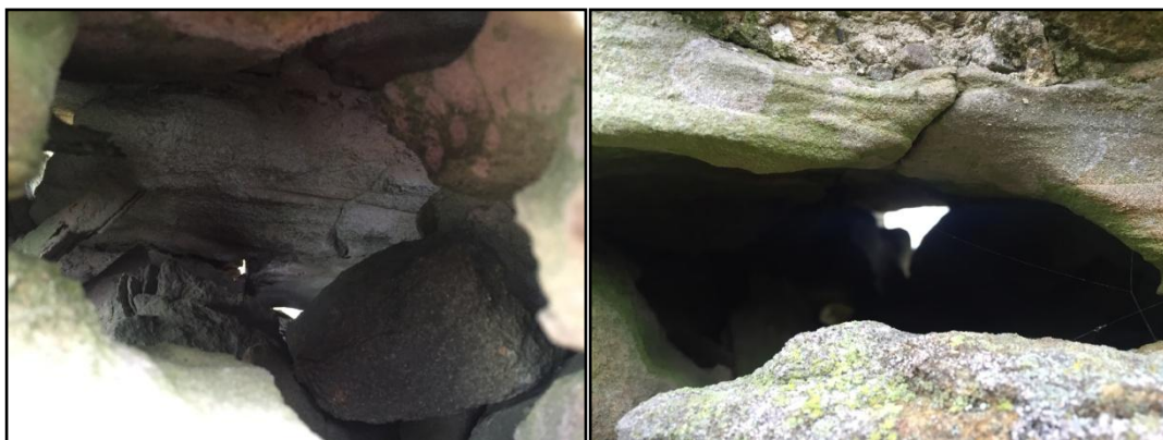
Figure 9. Large, open crevices within walls of main building.
