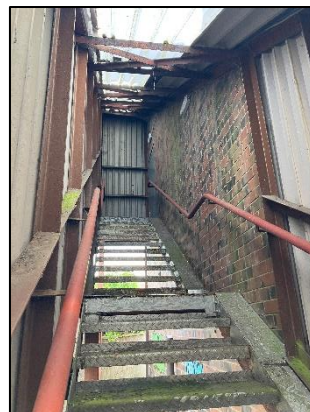
Figure 30: View up the redbrick and corrugated metal sheeting-encased fire escape on the western aspect of B1.
