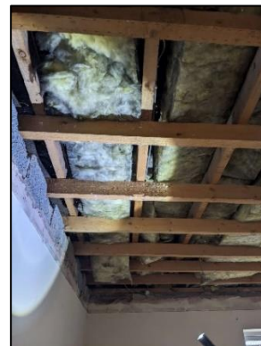
Figure 20: Exposed internal roof structure, indicating collapsed ceiling.
