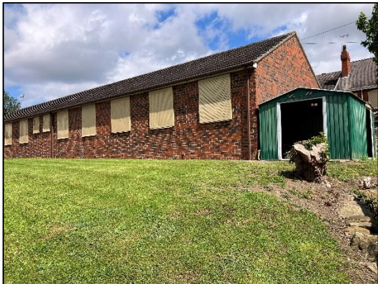
Figure 17: Single-storey extension on B1, view from the south of the site looking north.
