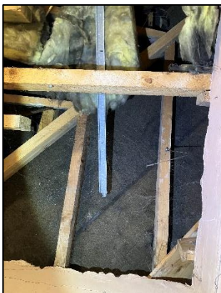
Figure 29: View of the internal roof structure – collapsed, revealing bitumen felt lining, similar on both structures.
