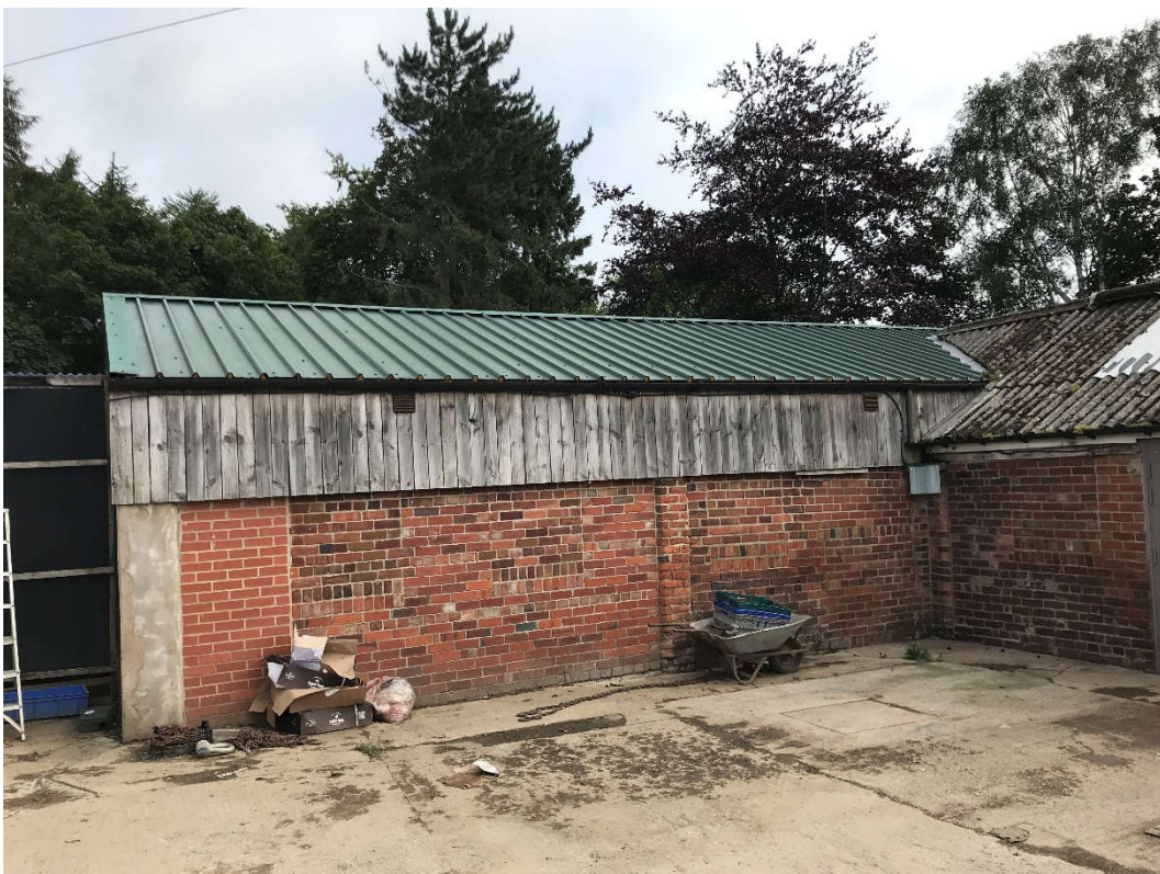
Fig 04. View of south elevation of Prep and Cold store building showing openings built up.
