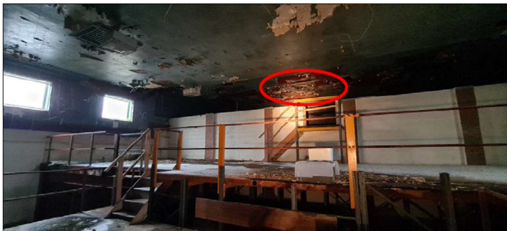
Plate 6. damaged ceiling with laths (circled red) visible
