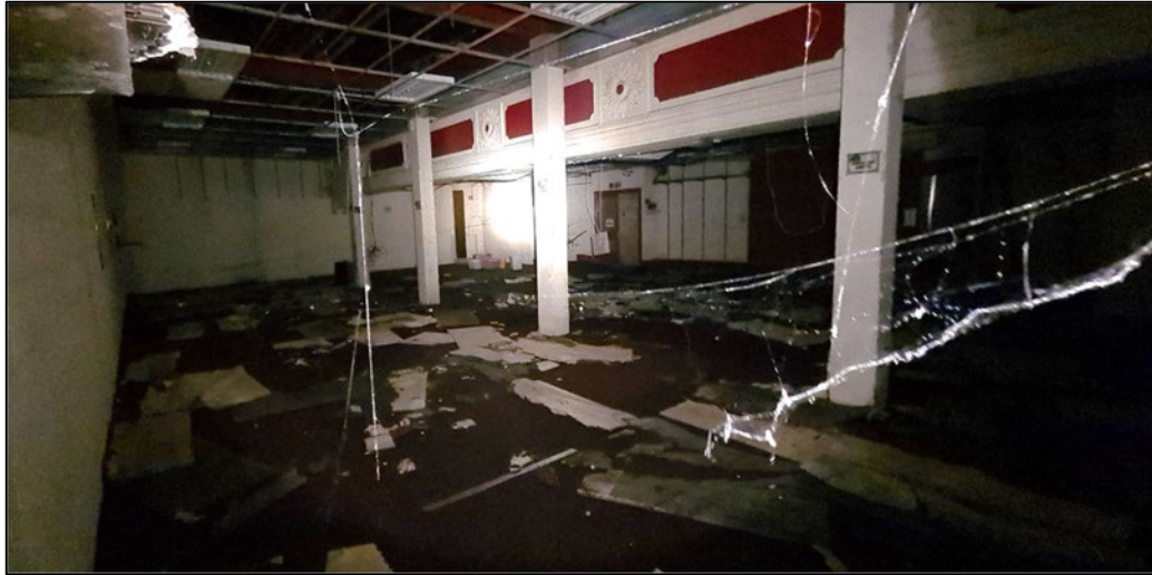
Plate 7. The foyer with very few suspended ceiling tiles remaining and hanging cobwebs shown
