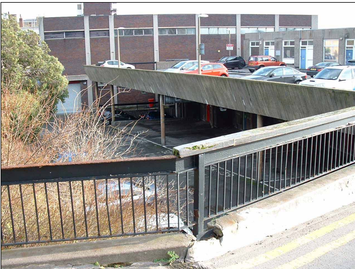
Plate 4. Two storey car park, north central area of the site looking east.
