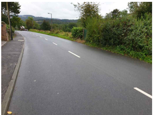
19 - Scarring and fretting on footway. Kerbs damaged and misaligned. Footway tarmac cracking and damaged
