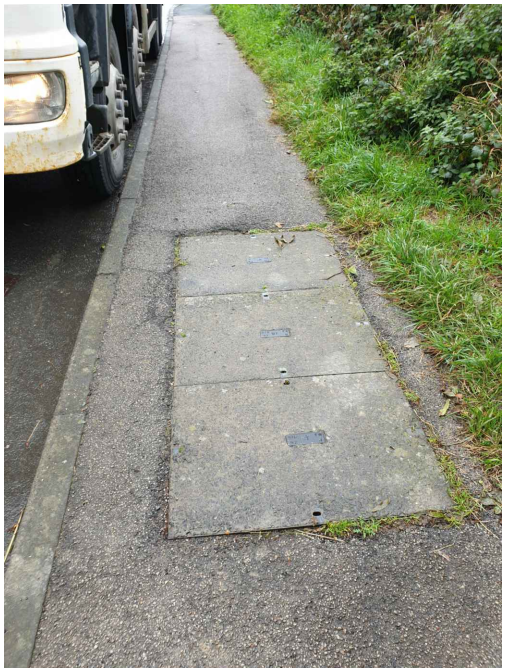
22 - Footpath around BT chambers badly damaged. Kerbs damaged and misaligned. Footway tarmac cracking and damaged
