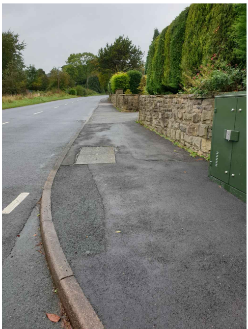
21 - Joint on junction is fretting. Kerbs damaged and misaligned. Footway tarmac cracking and damaged
