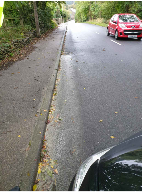
22 - Kerbs damaged and misaligned. Footway tarmac cracking.
