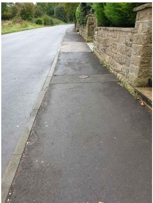
20 - Scarring and fretting on footway. Kerbs damaged and misaligned. Footway tarmac cracking and damaged
