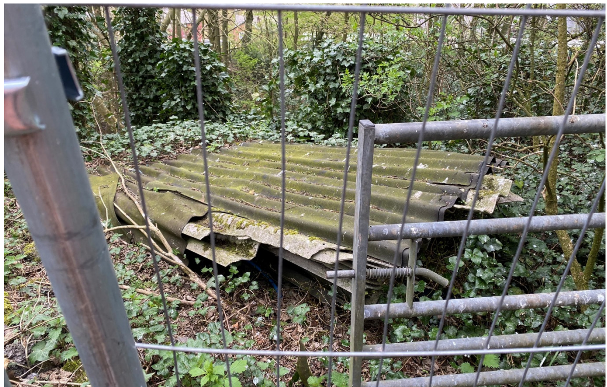
Photograph 4 – Stacked asbestos sheeting
