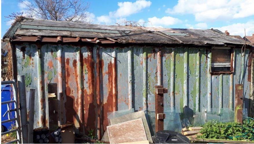
Photograph 1: Building B1 with gappy composite roof.
