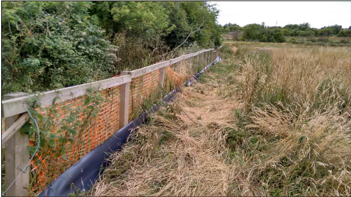
Plate 1: Photograph showing one-way herptile fencing located along the southern, eastern and western boundaries of the Site.
