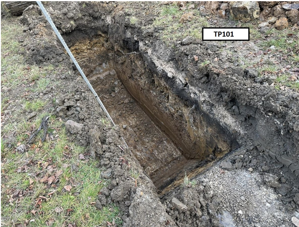
Photograph 03: Trial pit TP101. Southern side, eastern side, and base of trial pit. View from north west to south east.
