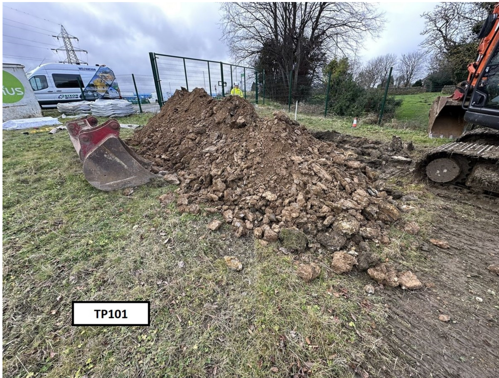
Photograph 05: Trial pit TP101. Trial pit arisings (2). View from south east to north west.
