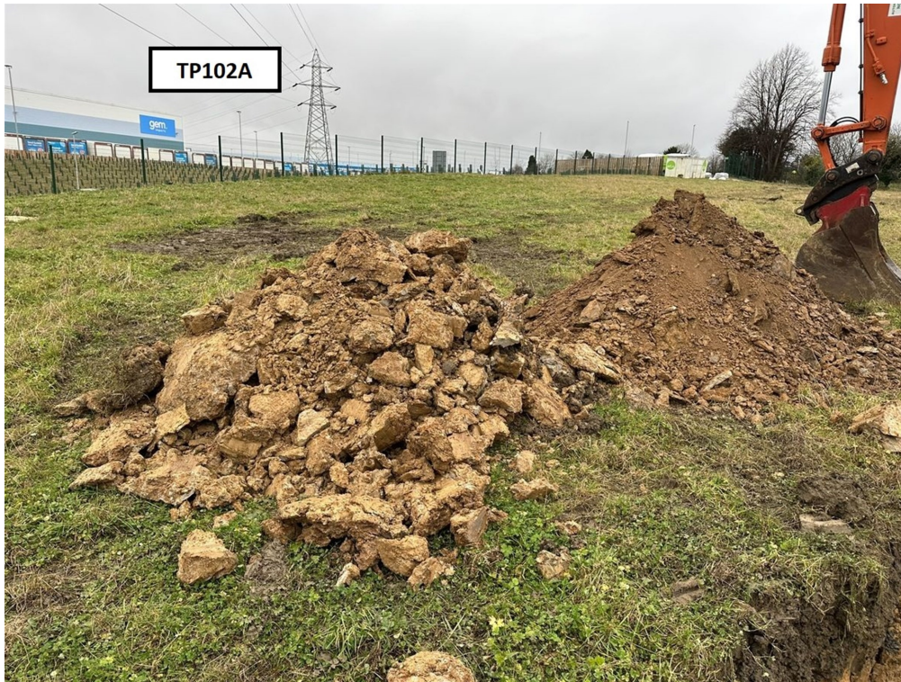
Photograph 10: Trial pit TP102A. Trial pit arisings (2). View from south east to north west.
