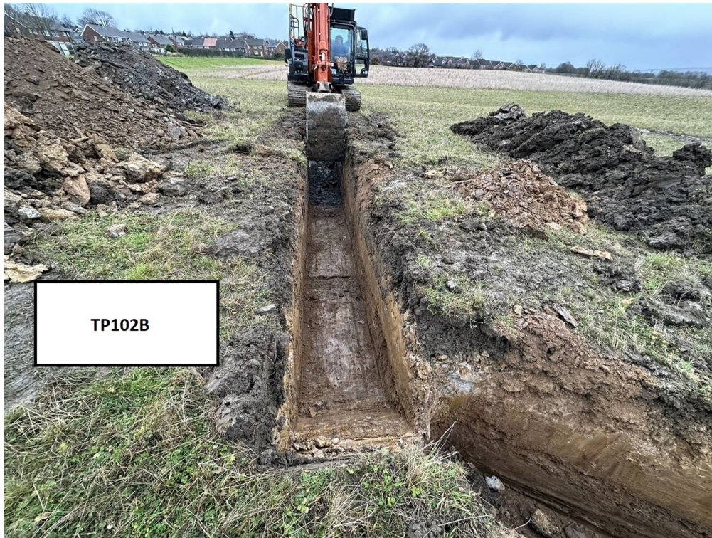
Photograph 11: Trial pit TP102B. View of trial pit while excavation is ongoing. View of trial pit from south west to north east.
