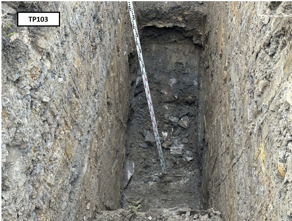
Photograph 19: Trial pit TP103. Base of trial pit. View from east to west.
