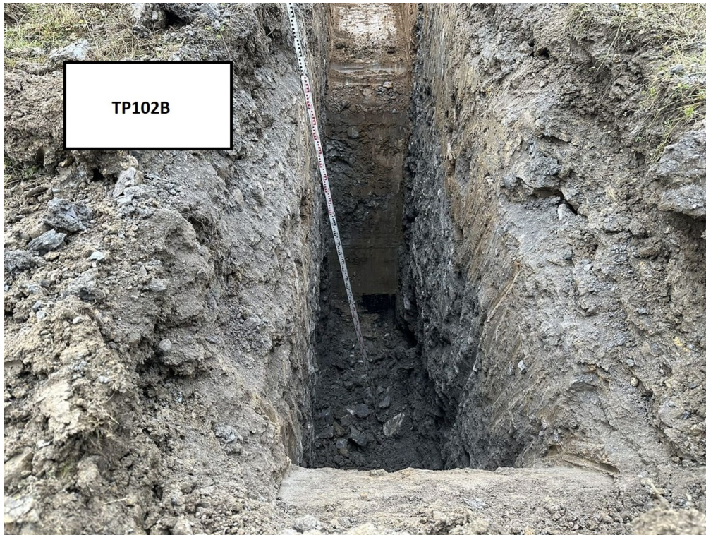
Photograph 13: Trial pit TP102B. High wall of opencast mine workings identified in the central pit area. View from north east to south west.
