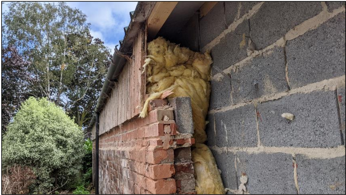
Plate 10. Collapsed section of brickwork on north elevation of outbuilding
