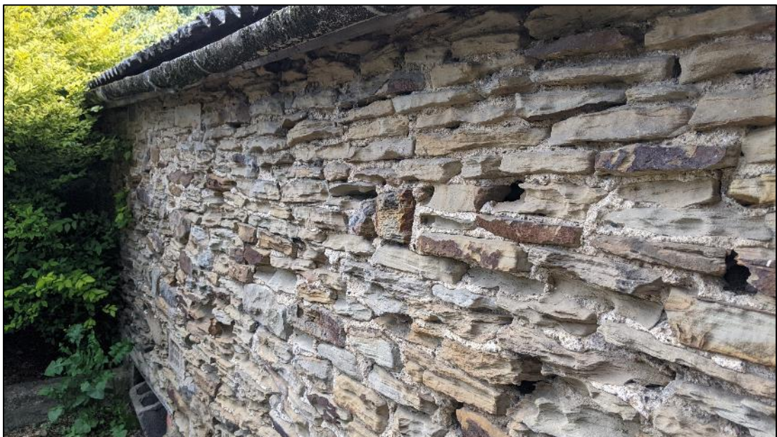
Plate 9. Dry and dusty hollows in stone wall on east elevation
