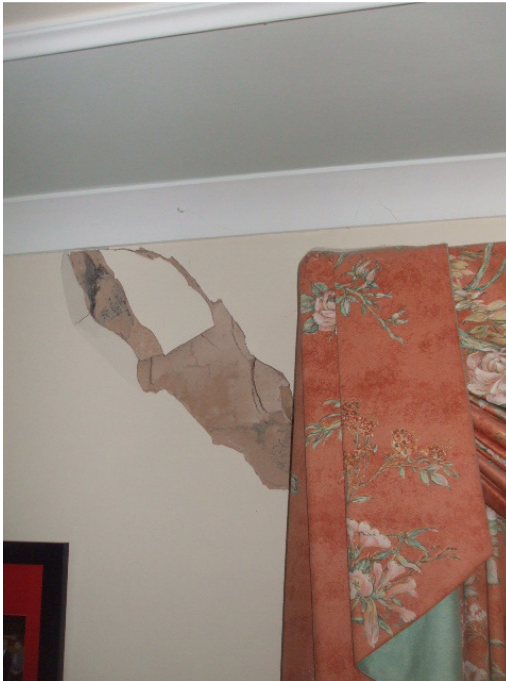
Cracking and de-bonded plaster to left-hand side of window in front left-hand bedroom.
