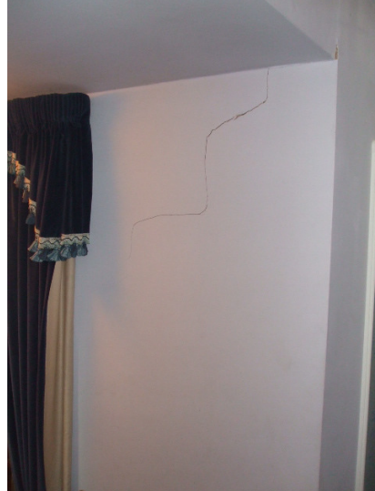
Cracking in hallway link / study area.
