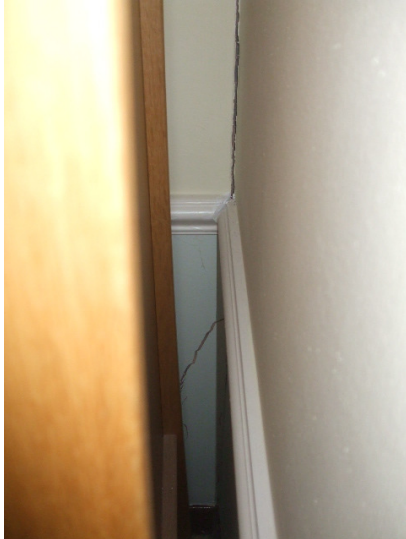
Cracking to left-hand wall in front right-hand bedroom.
