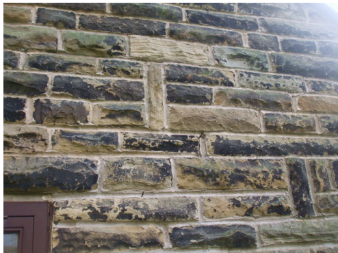
Stepped cracking to front elevation.
