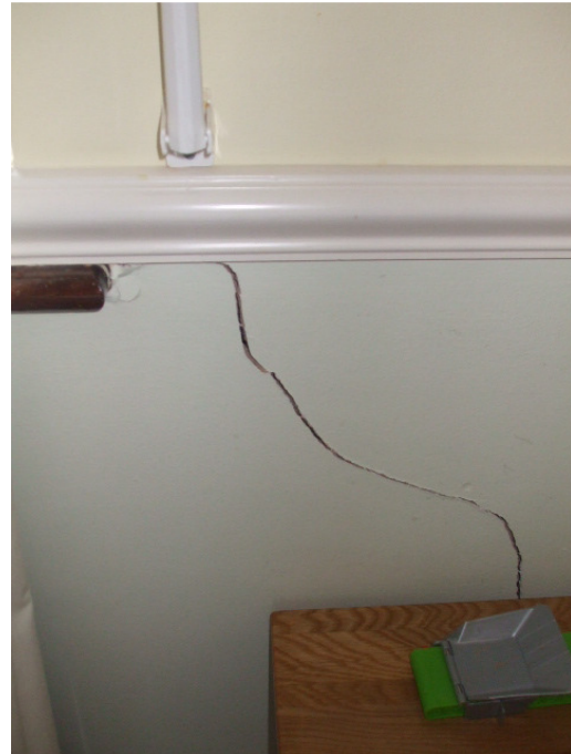
Cracking to bottom right-hand corner of window in front right-hand bedroom.
