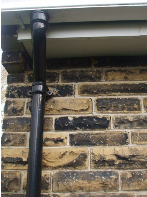
Stepped cracking to right-hand wall of front right-hand projection, where the front right bedroom is located.
