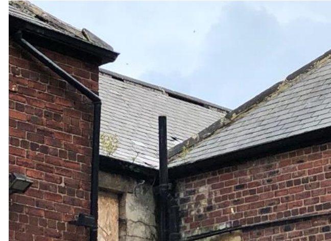
A smaller area of missing tile and gaps along the roof ridge
