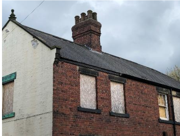
Area with missing guttering
