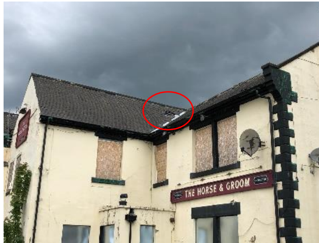
Area of missing tiles in the roof
