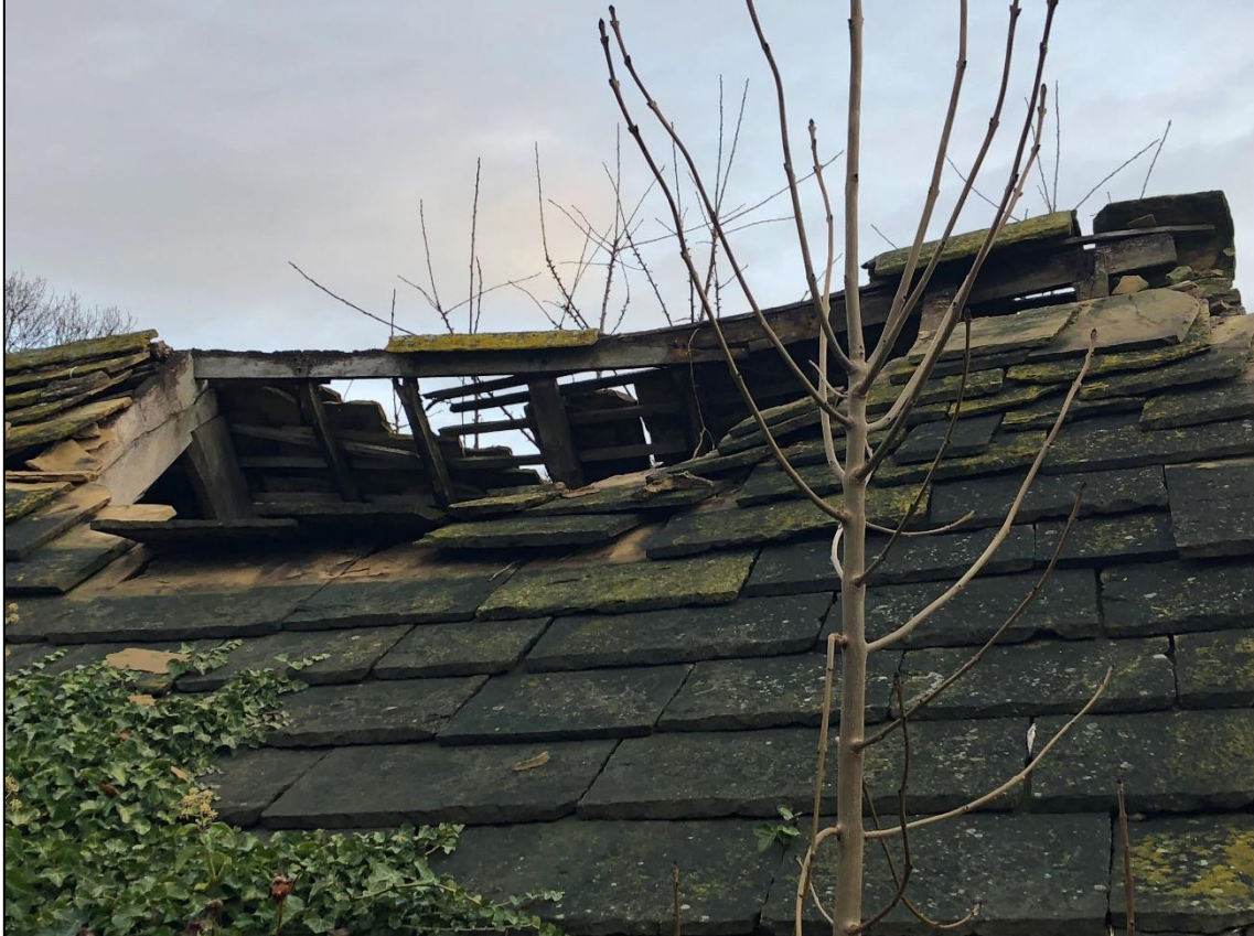
Figure 10: The collapsed section of roof.
