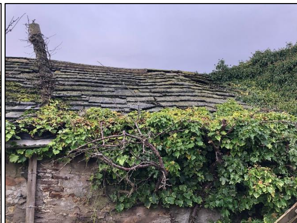
Figure 12: Showing the poor condition of the roof.
