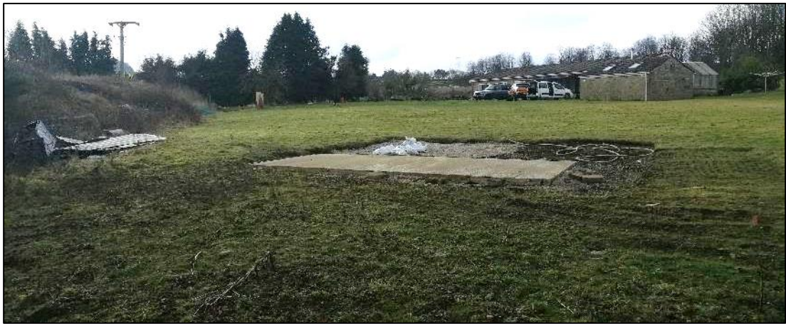
Plate 5. Concrete pad and unsealed surface with gc3 on left (bund) and in foreground
