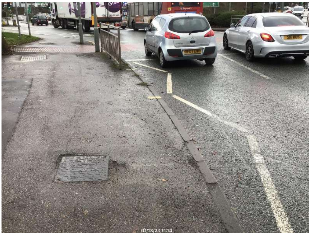
24) South Tie in East footway: low failed tarmac around chamber
