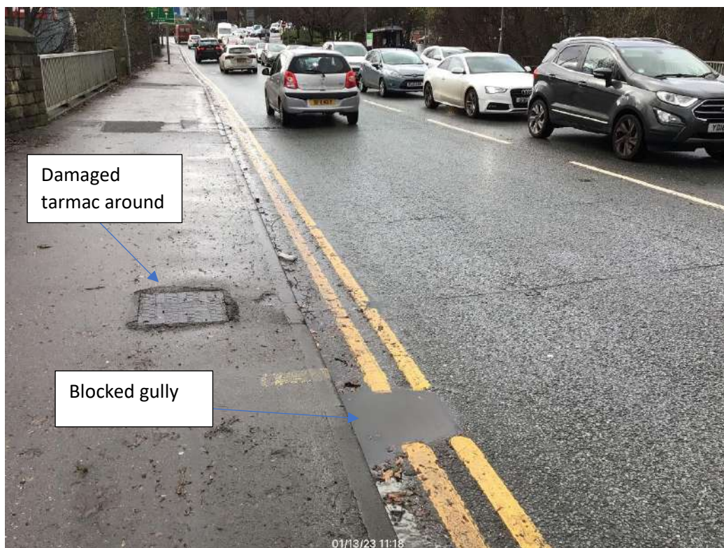
36) North of bridge, Southbound Lane: Blocked gully & damaged tarmac around chamber in footway
