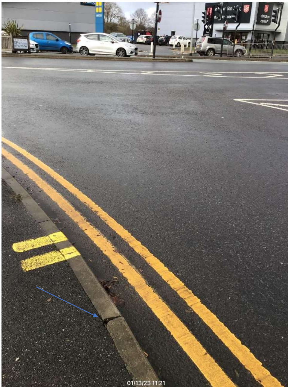
42) Northeast tie in, East kerb line: damaged kerb
