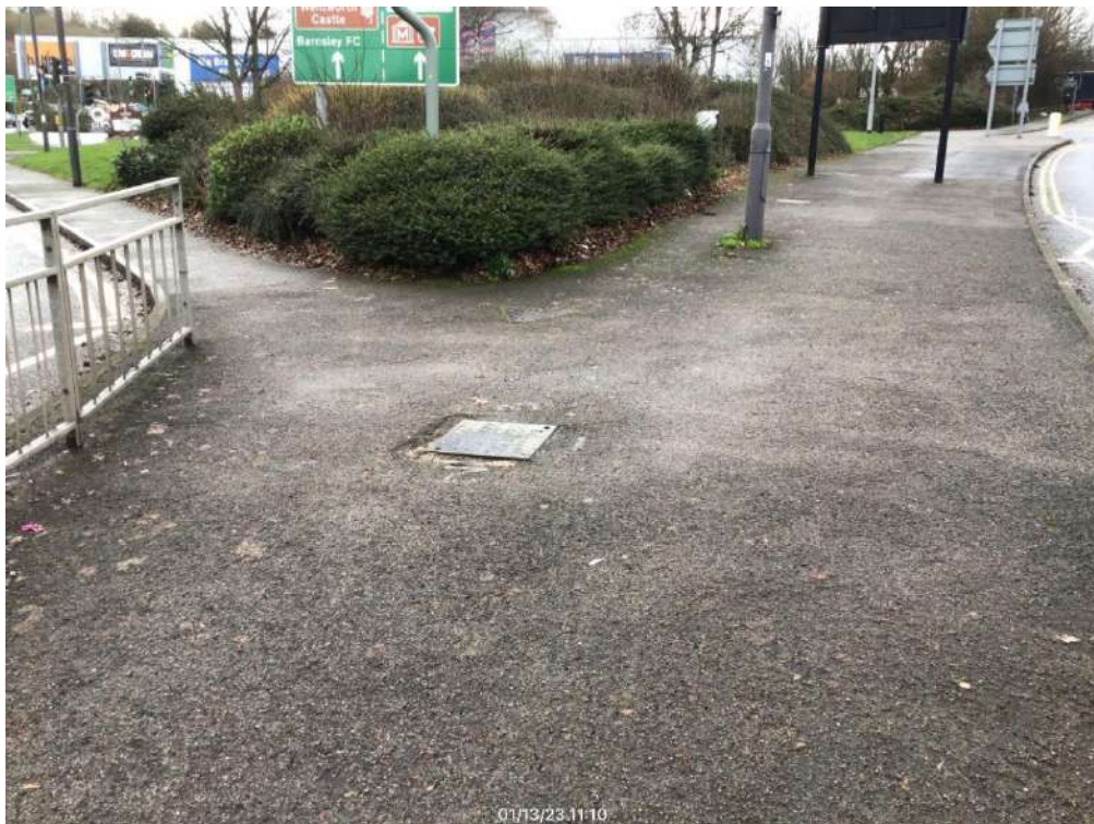
21) South tie in island: low/sunk tarmac surround around chamber
