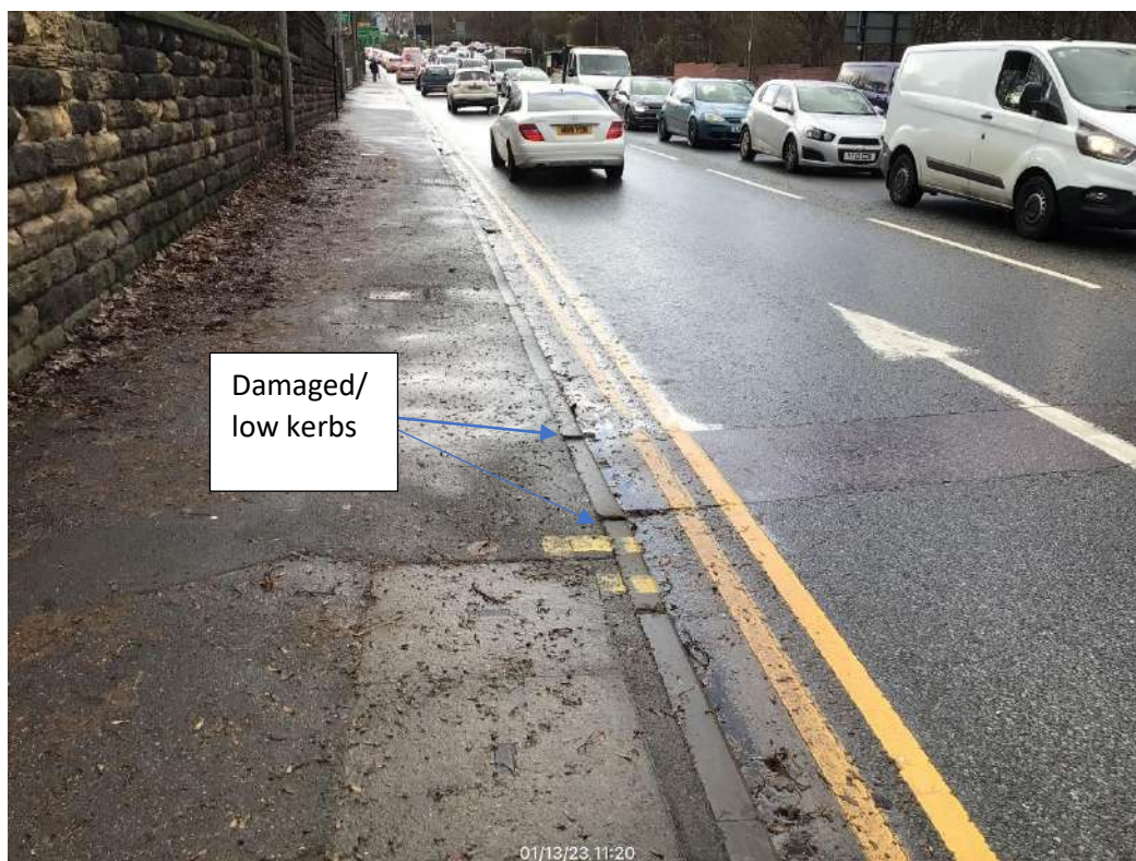
41) North of bridge, Southbound: Damaged/low kerbs from trench reinstatement works
