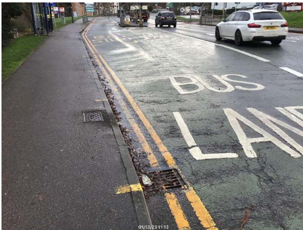
22) South tie in, Southbound bus lane: Cracking to bus lane surfacing & blocked gully
