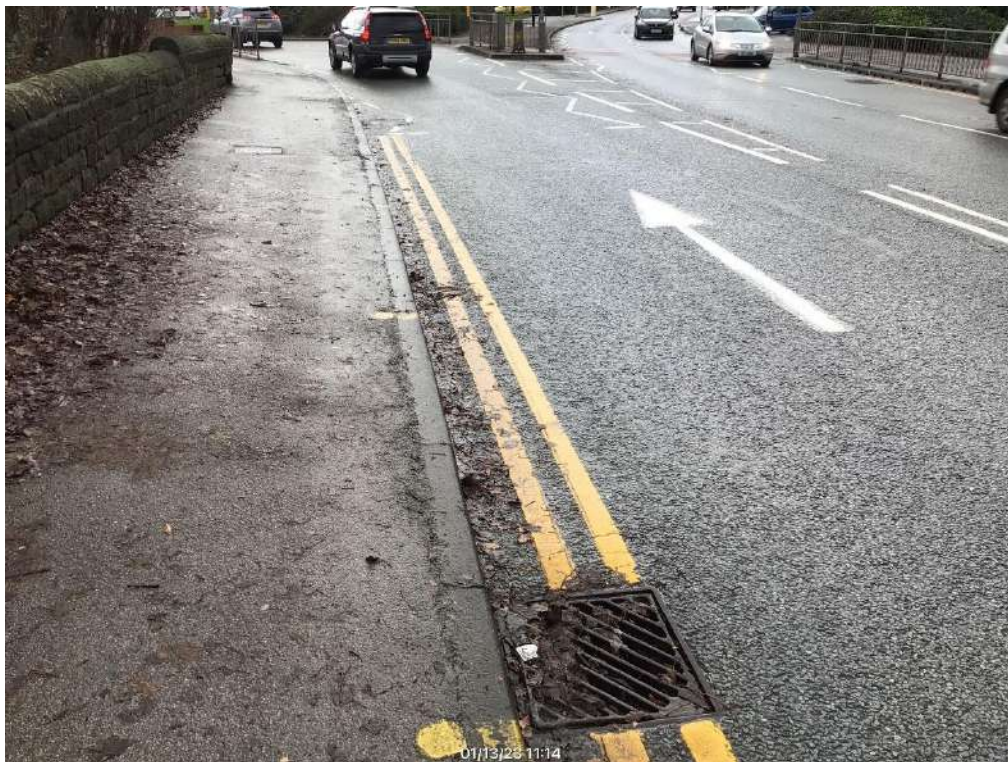
27) South of bridge, Southbound: Blocked gully
