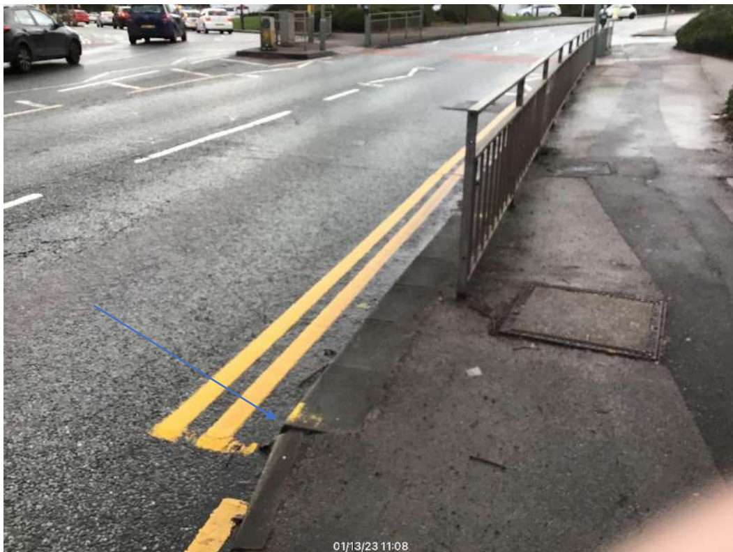
18) South of bridge Northbound/Bus lay by taper: Damaged kerb
