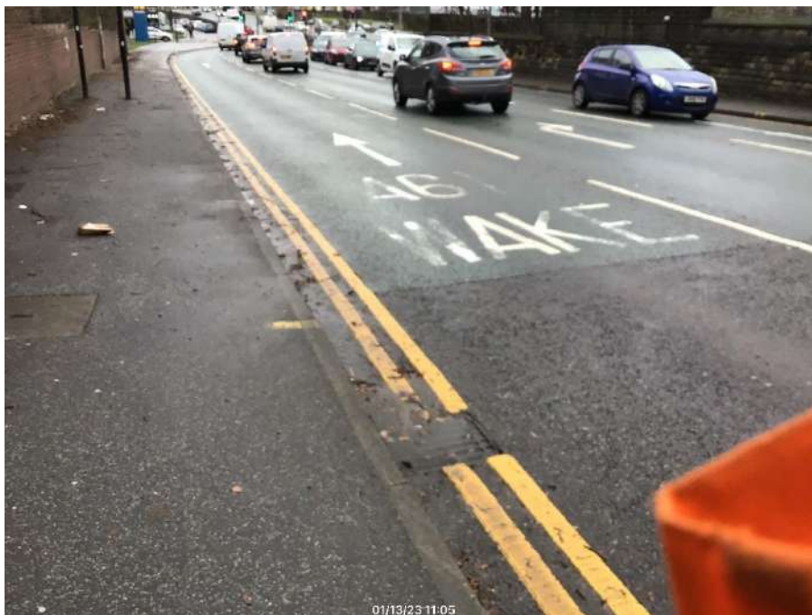
10) North of bridge, Northbound: Blocked gully
