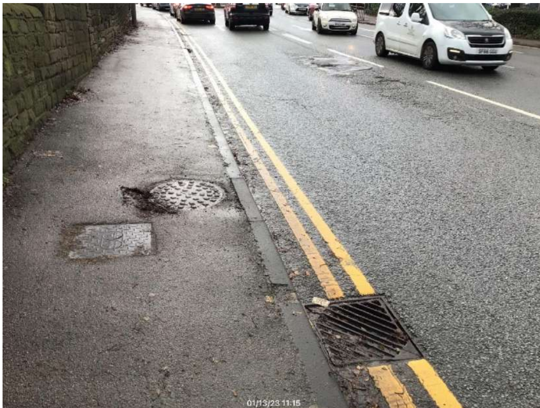
29) South of bridge, southbound: Blocked gully
