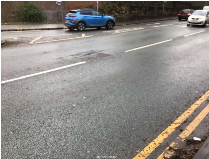
7) Northbound Lane 2: Low chamber with surrounding surfacing course damage
