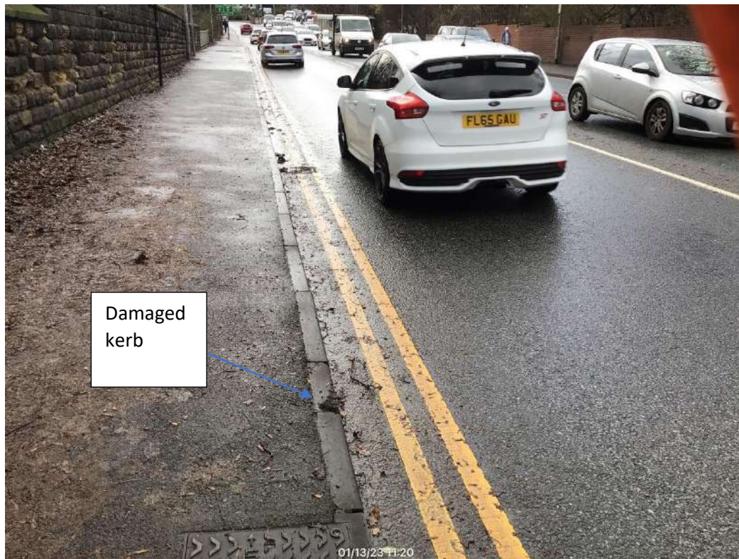
40) North of bridge, Southbound: Damaged kerb
