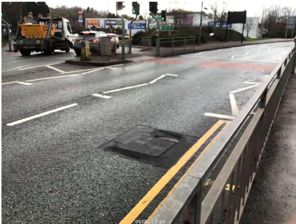
19) South of bridge, Northbound Lane 1: Damage to surfacing around chamber
