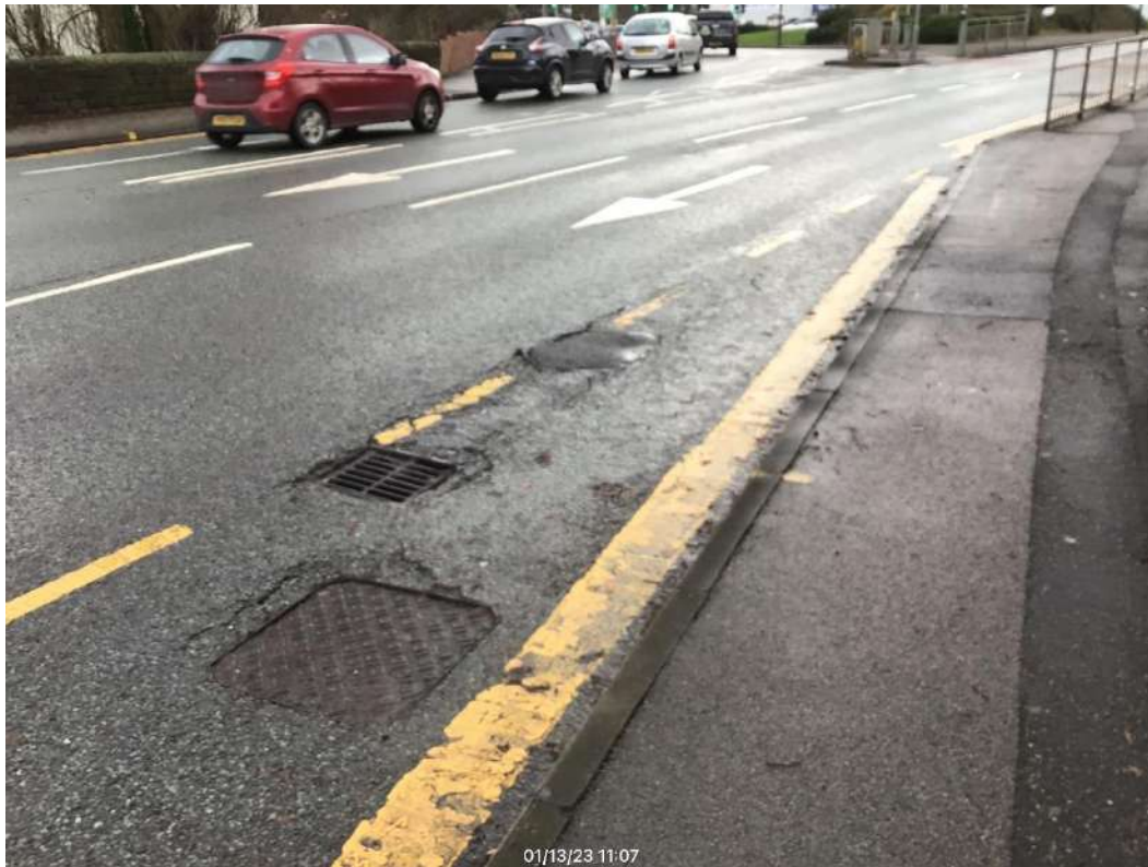
17) South of bridge, Northbound Bus stop taper: failed/cracking to surface course around chamber & gully
