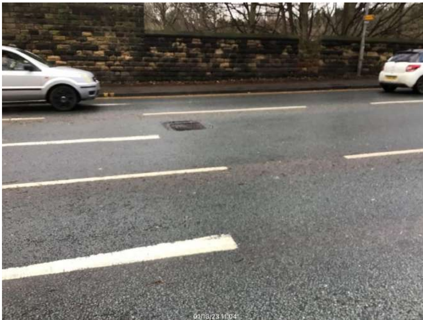
8) Northbound Lane 2 low chamber with surrounding surfacing course damage
