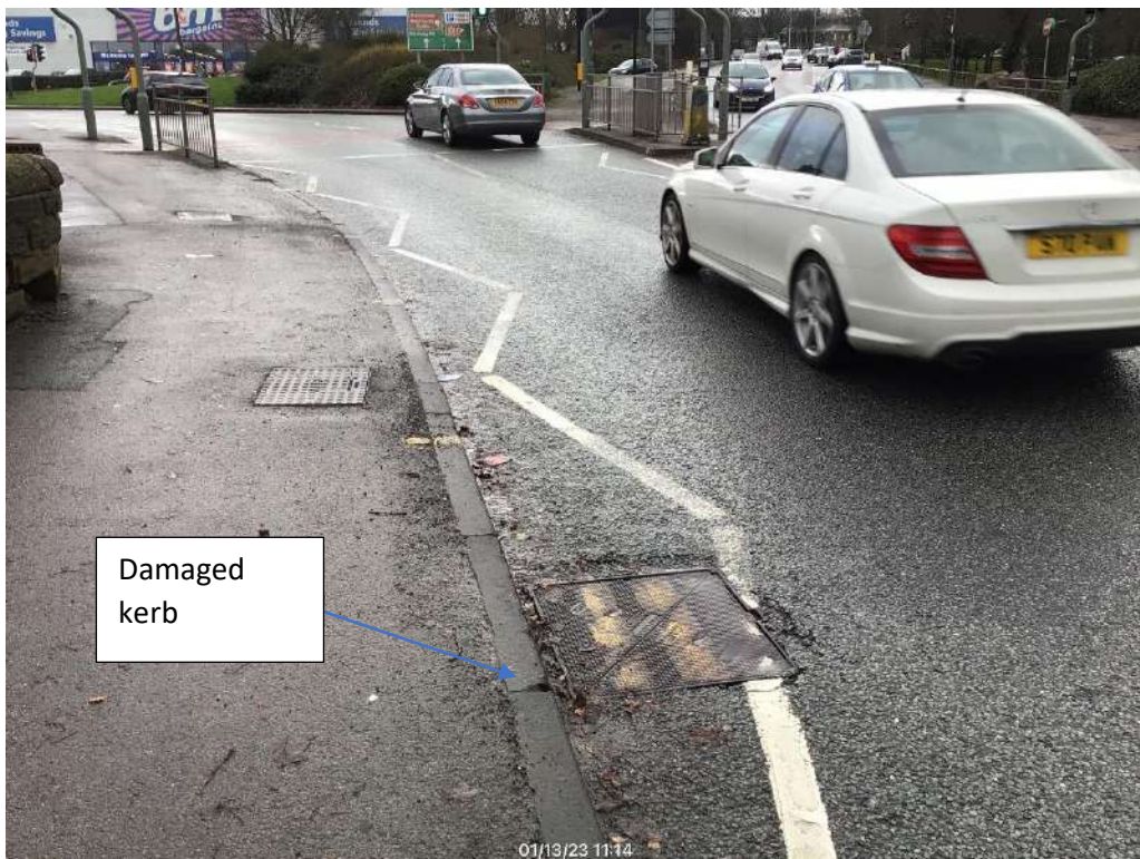
25) South tie in, Southbound: damage to kerbs
