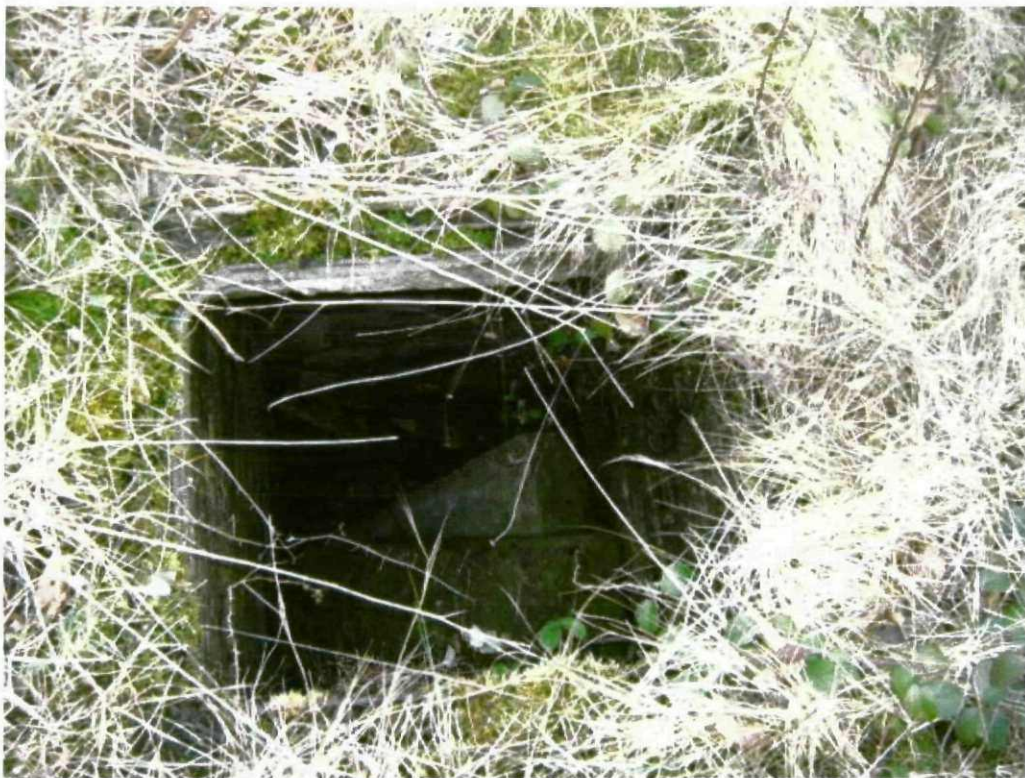
Photograph number 28 showing the same inspection chamber with debris inside.
