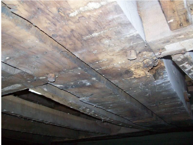
19 Cracks through the second principal beam
