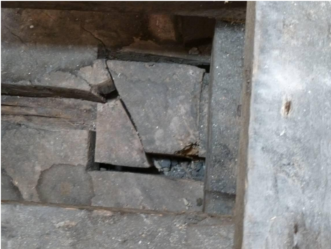
9 (Failed) wedge at south end of historic repair
