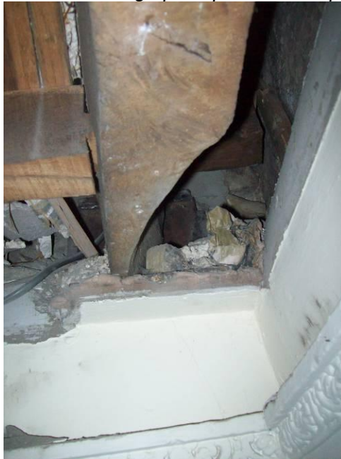
17 Secondary beam end barely bearing on the masonry at western wall
