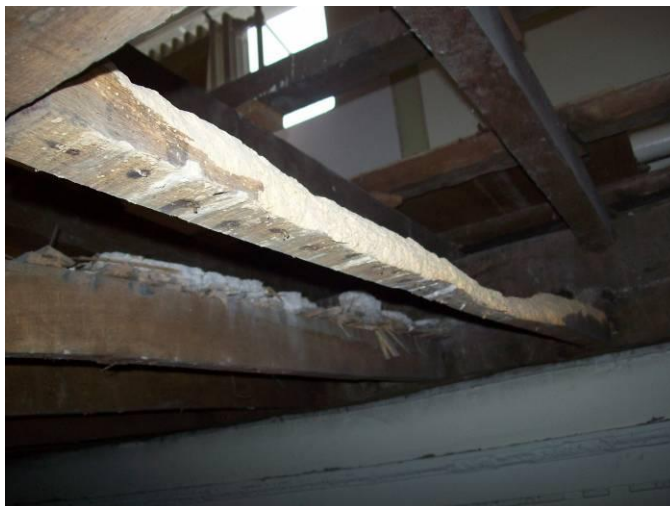
18 Ceiling joists eaten away by beetle attack
