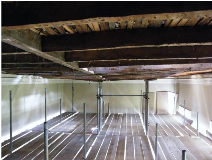
21 View of the underside of the propped floor structure showing the severity of the deflection in relation to the wall frieze
