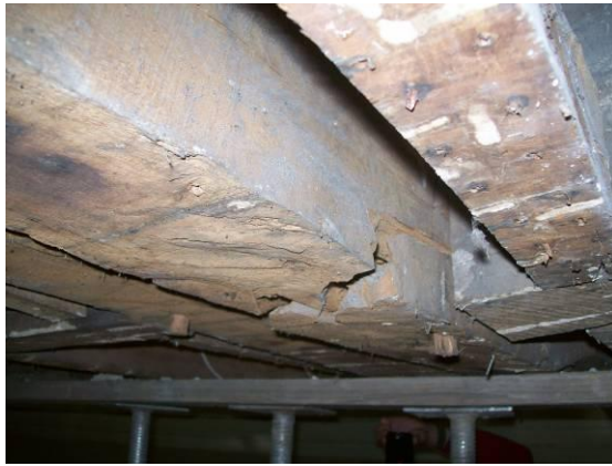
16 crack through principal beam requiring scaffold propping
