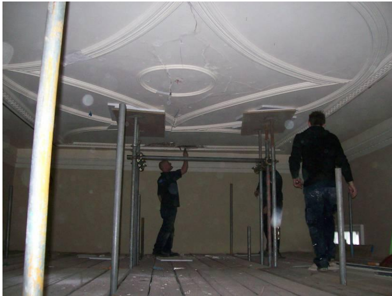
15 propped ceiling showing mid line cracking and deflection
