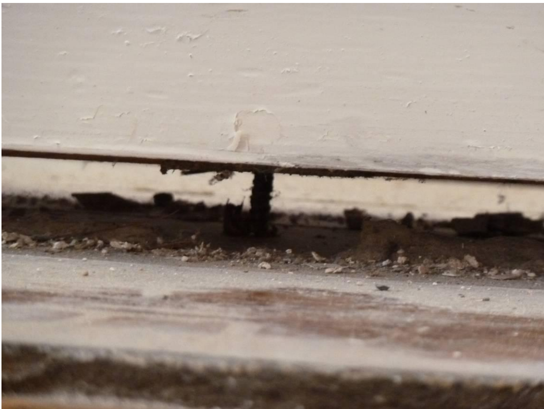
3 Second floor structure settling below the second floor partitions pulling screw fixing of partition sole plate away June 2011
