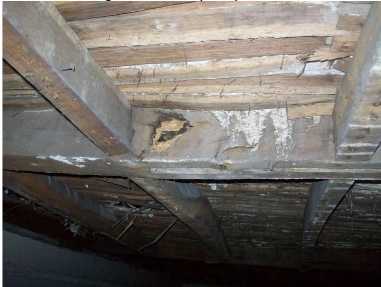
20 Deep pockets of soft crumbling decayed wood in secondary beam
