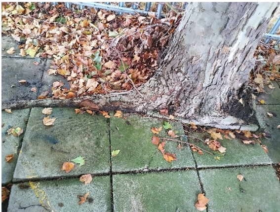
Photo 7: T7 pavement damage
