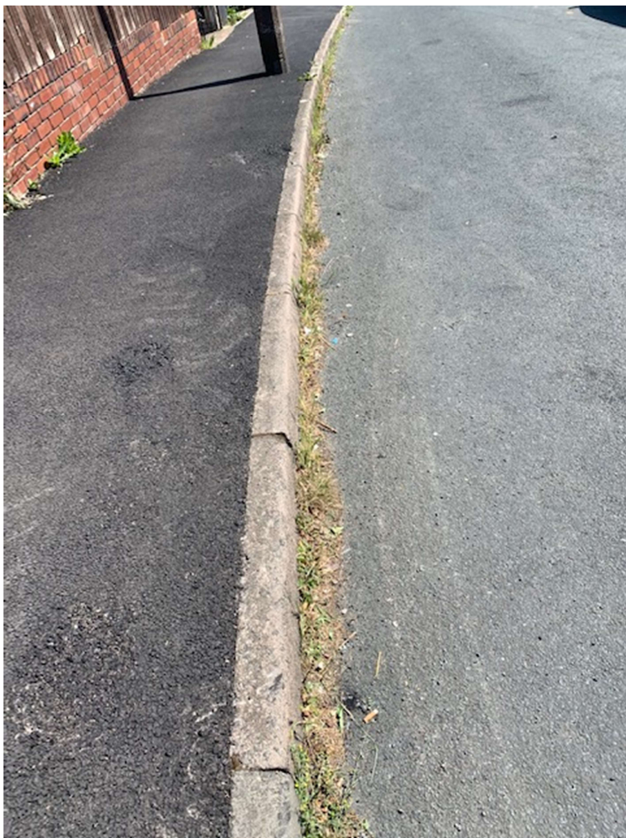
Kerb / footpath opposite site entrance on Heysham Green
