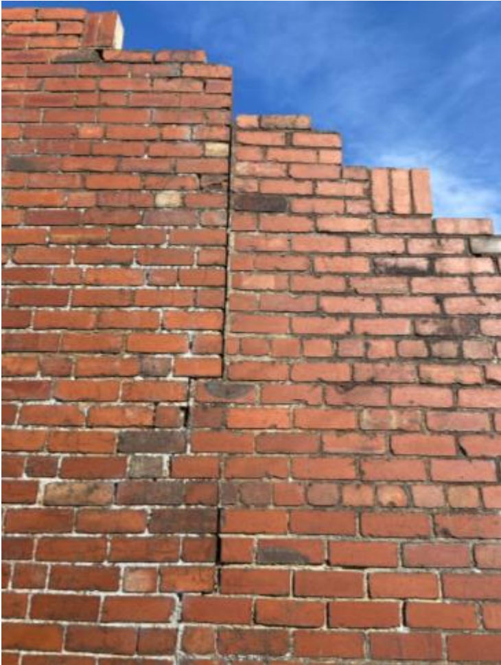
Photo P1B – Cracking to Gable End
