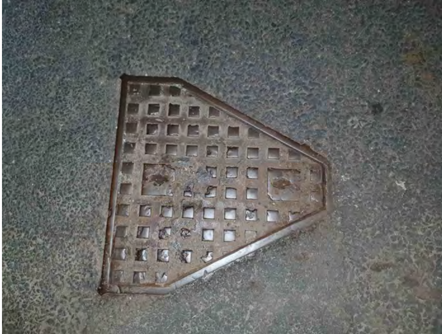
CW4 UTR Cover Stuck
