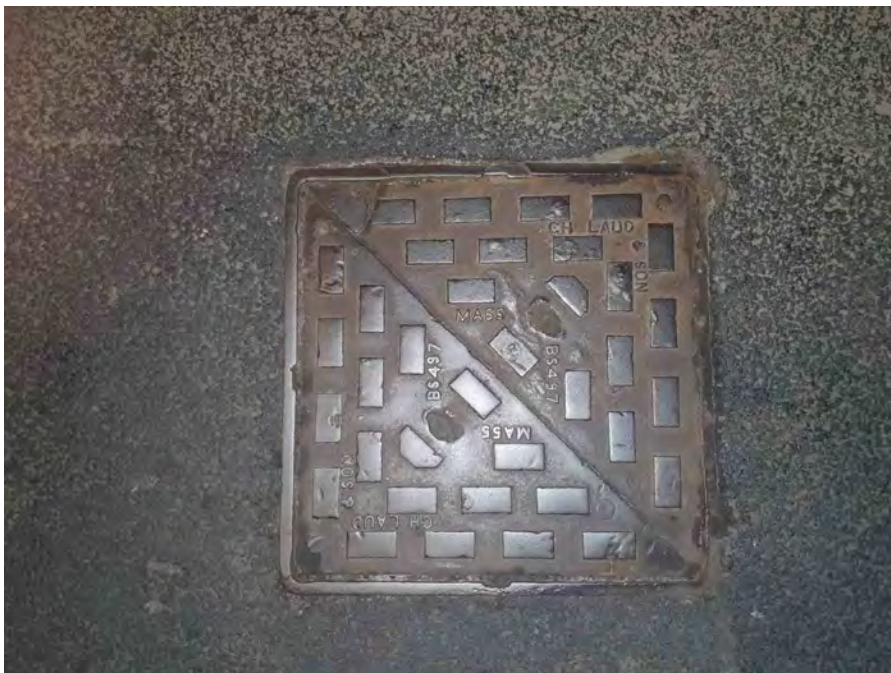
Mh3 UTR Cover Broken
