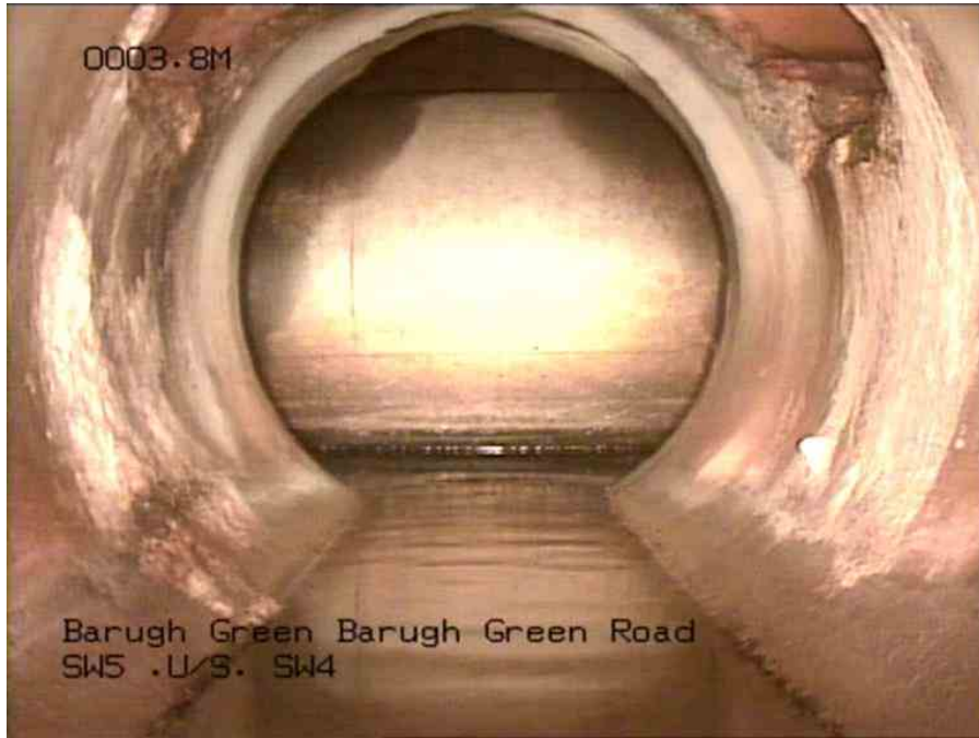
1, 00:00:31, 3.80 m Hole in drain or sewer from 11 o'clock to 1 o'clock
