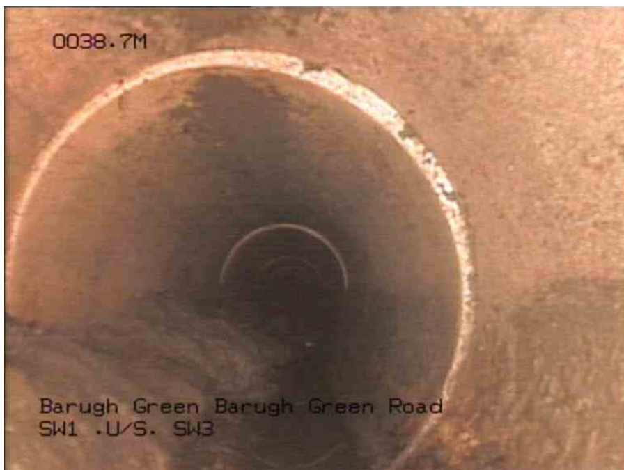
2, 00:05:35, 38.70 m Settled deposits, other, 20% cross-sectional area loss, Mud
