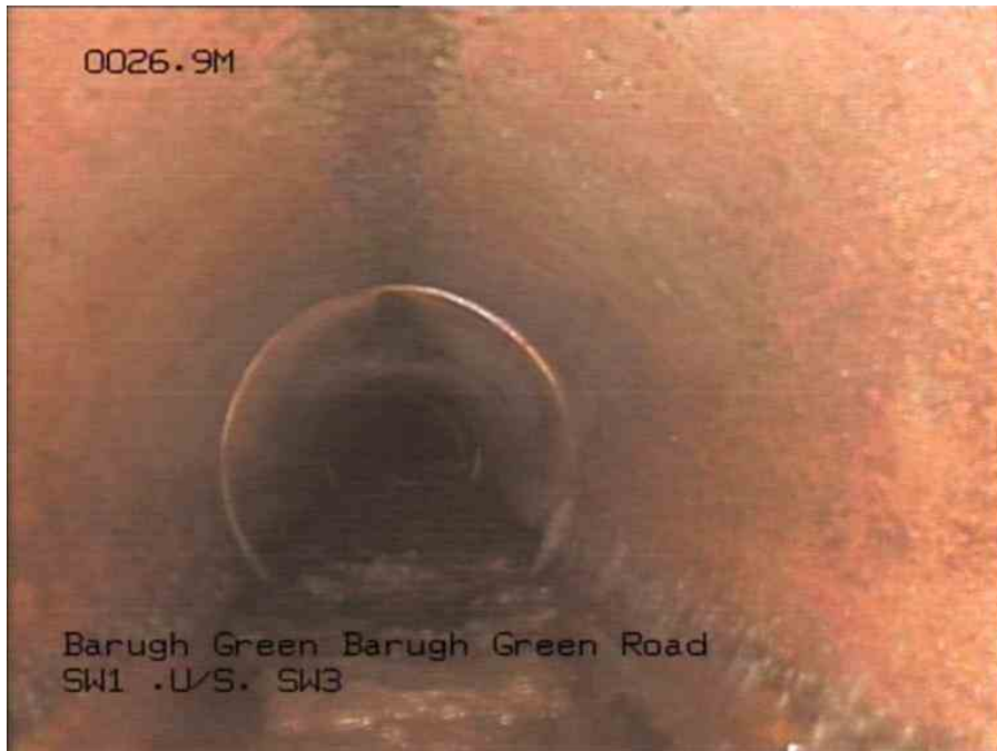
1, 00:03:00, 26.90 m Settled deposits, other, 15% cross-sectional area loss, start, Mud
