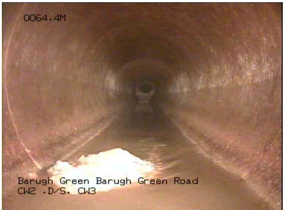
2, 00:03:42, 64.40 m Settled deposits, other at joint, 10% cross-sectional area loss, Rags
