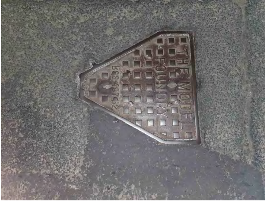
CW1 UTR Cover Stuck
