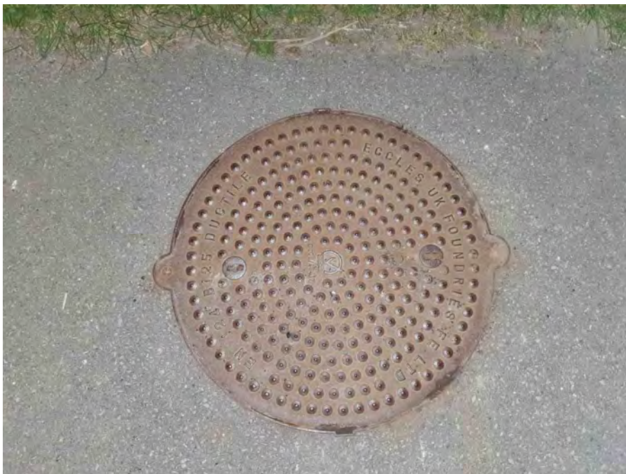
SW2 UTR Bolted Cover Seized
