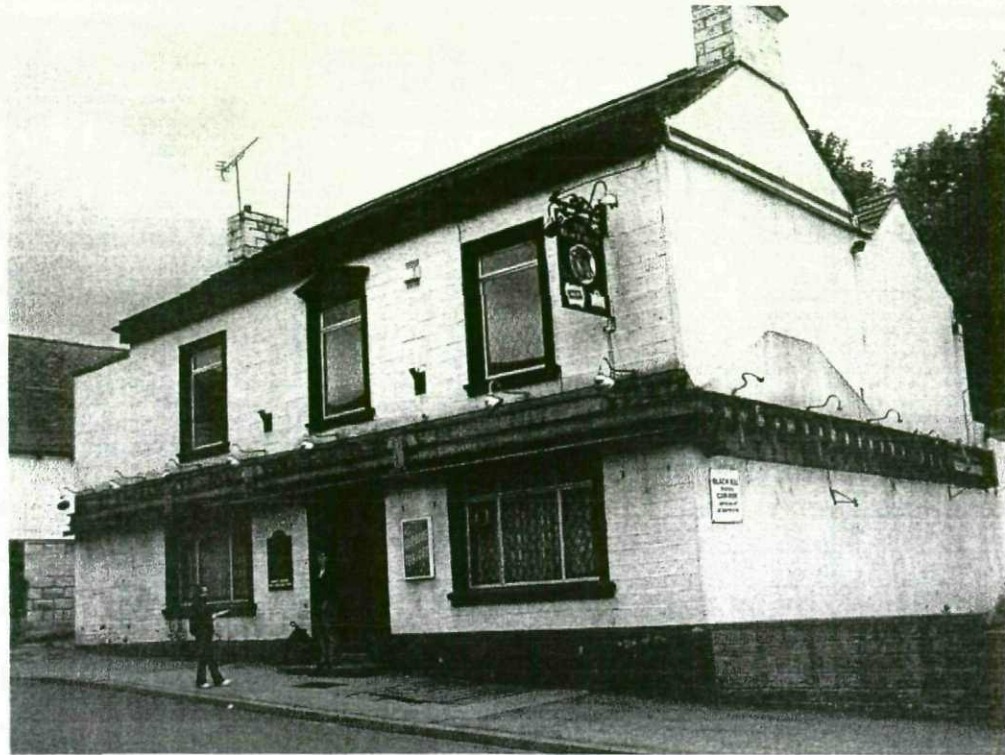
Plate 1 Main elevation to Manchester Road showing steel strapping at first floor and eaves level
