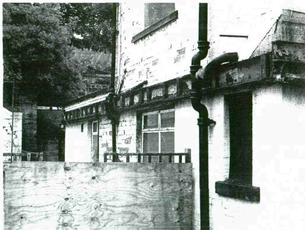
Plate 4 West side gable strapping at first floor and extending full length to include single storey extension added later
