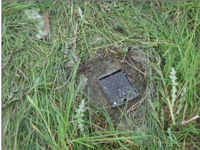
Photo 7: WS01 – Lockable metal cover to gas monitoring installation.
