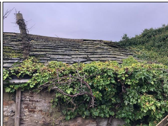
Figure 12: Showing the poor condition of the roof.
