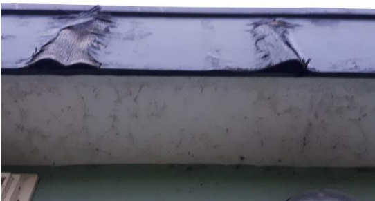
Photograph 8: B1 (delaminating fascia)
