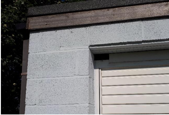
Photograph 10: B3 (gap above door)
