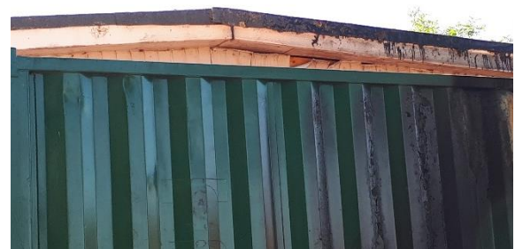
Photograph 9: B2 (damage to gable)
