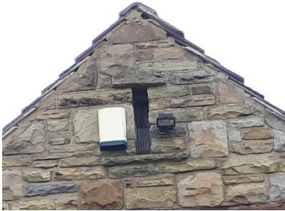
Photograph 12: B6 (hole in gable end)
